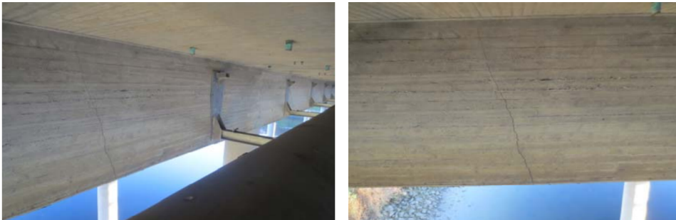
Figure 4.6: Cracks appearing at the original zero moment section between axis 8-9, 4,5m after axis 8. (Aas Jacobsen, 2013)
