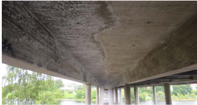
Figure 4.9: Picture taken at axis 1 showing the western side of the bridge deck (Aas Jacobsen, 2013).
