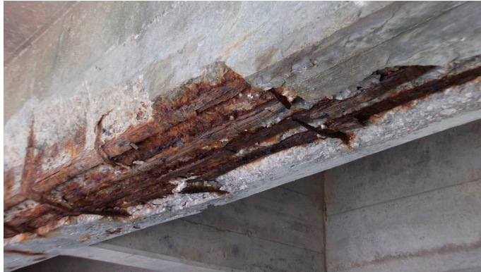
Figure 3.2: Spalling due to voluminous corrosion products
