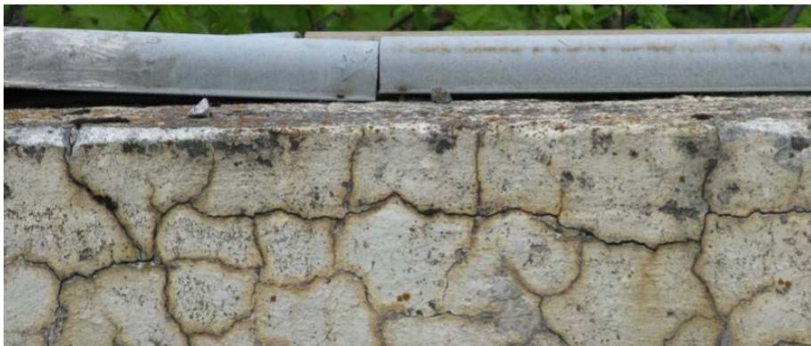
Figure 2.4: ASR - map cracking at railway bridge in Trondheim
