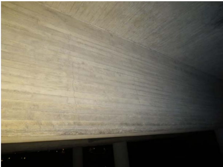
Figure 4.8: Typical cracks occurring in the field sections. Closed in bottom and top. (Picutre taken between axis 5-6) (Aas Jacobsen, 2013)
