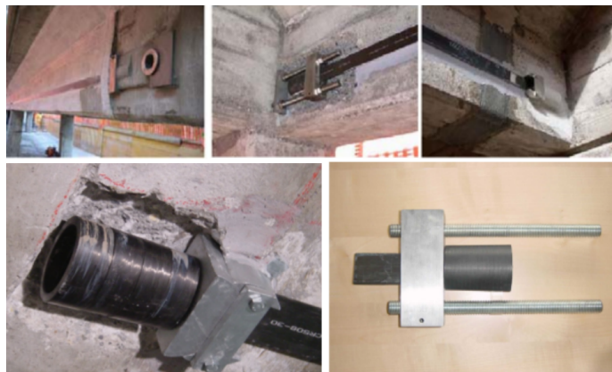
Figure 4.13: Test project using carbon fiber strengthening at inner beams. Glued to the beams with epoxy. Mechanical anchor at ends (Aas Jacobsen, 2015)
