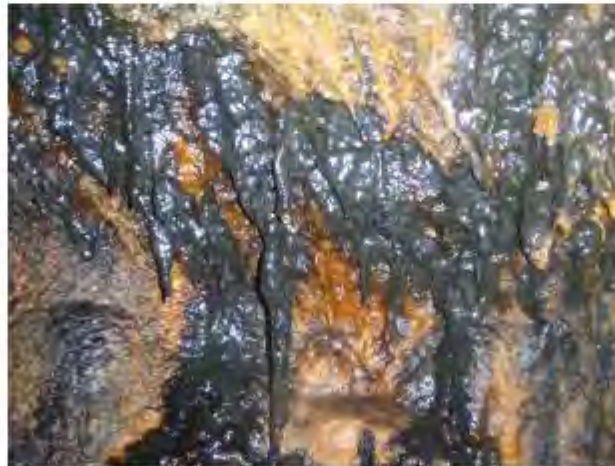
Figure 2: Example of sprayed concrete degradation at the Oslofjord Test Site before it was established. Calcite stalactites were covered by dark Mn-bacterial slime and rusty Fe-bacteria. Concrete underneath was friable. Width of field about 40 cm.
