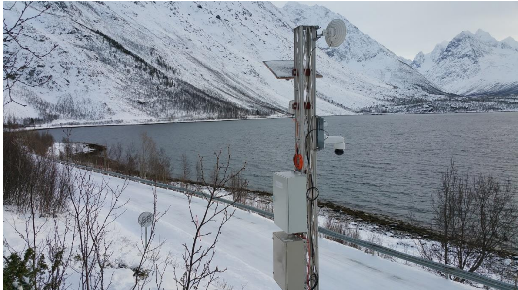
Figure 3: Radar system on the day of installation (17 February 2017).
