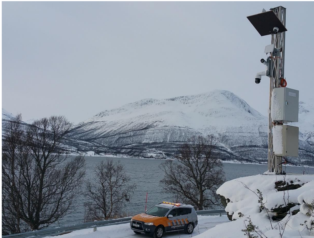
Figure 2: Radar system on the day of installation (17 February 2017).
