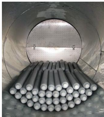
Figure 16. PCM rods placed inside a water tank.
