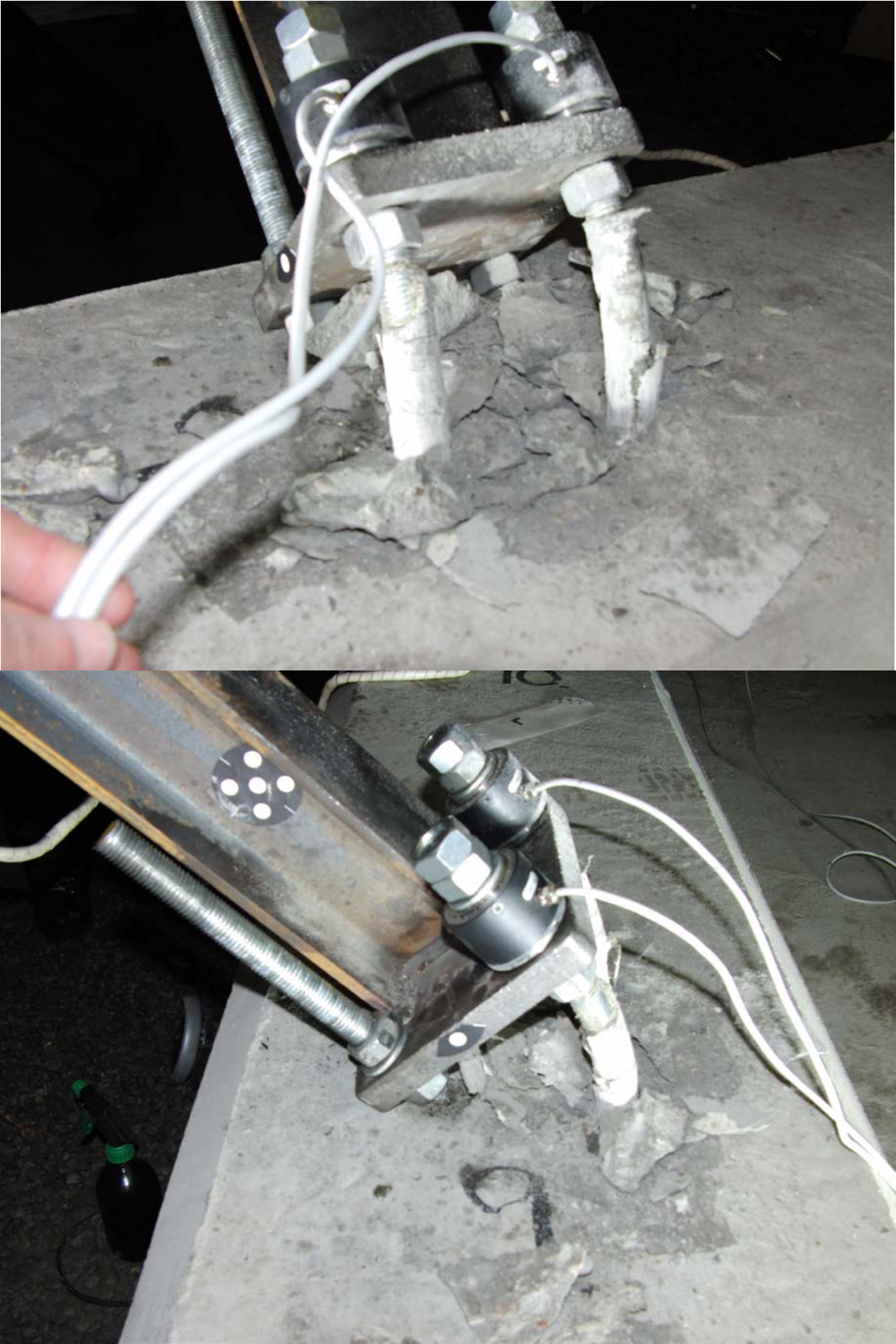
Figure 3 – Failure of the chemical anchorages
