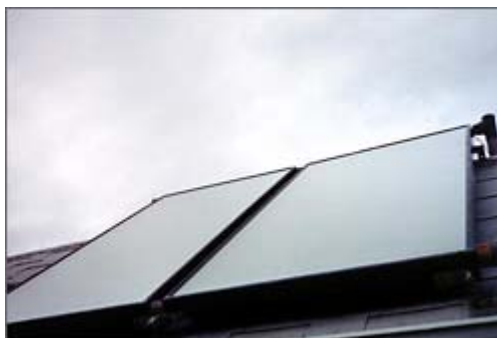
Photography 2.2.3.II. – Solar hot water equipment for a building.
