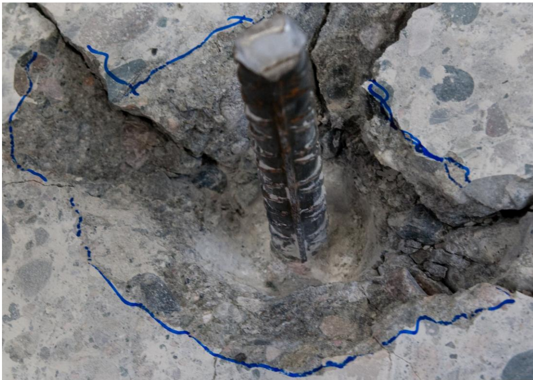
Figure 7-8: Crater made by the shoe with the concave end face with predrilling, test series 3
