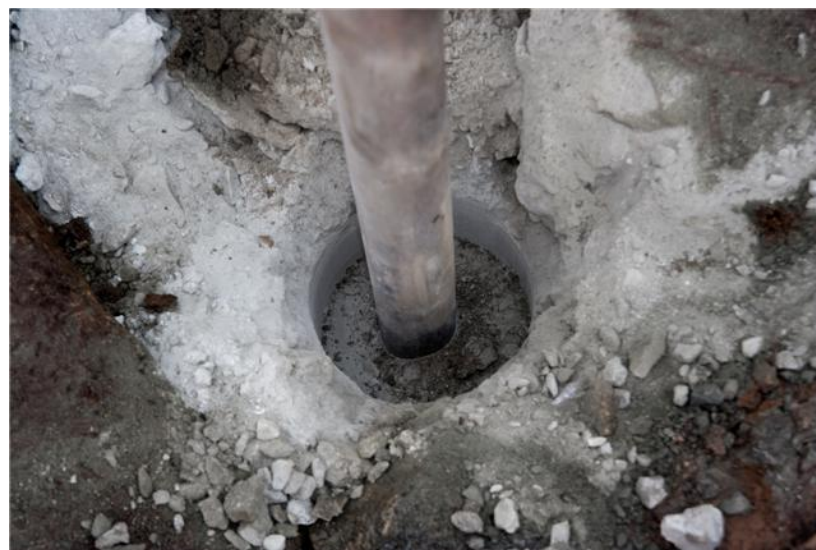
The rock after Shoe no. 1 has been chiselled in and then extracted.
