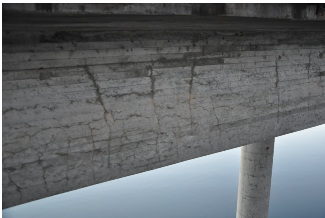
(a) Krakeleringsriss i bjelke
