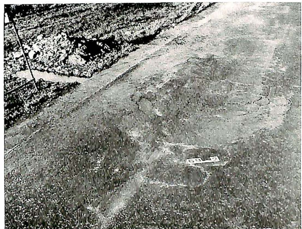
Fig. 12. Surface of an area on Section 69 at Alconbury Hill, after 2½ years, shortly before reconstruction.
