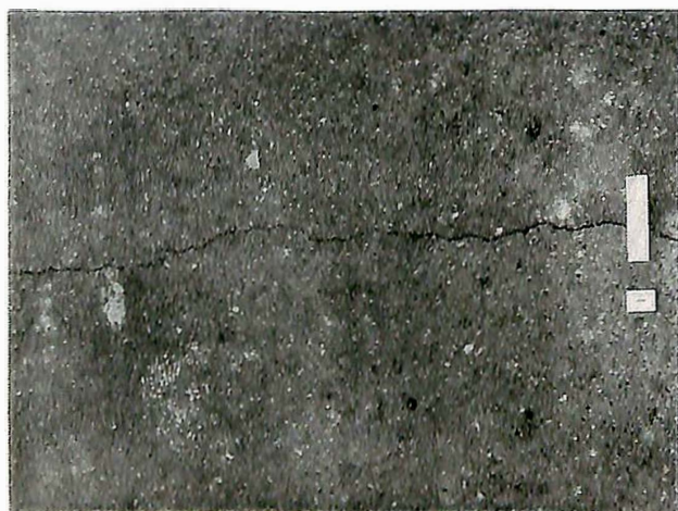
14. Typical transverse crack in bituminous surfacing over a lean concrete base.
