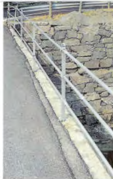
Figure 12.3 Steinhvelvs Bridge, Søndeled, Aust Agder. Several layers of asphalt, which have not been smoothed down, form uneven, horizontal edges. The road surface is now higher than the bridge's original level. The uneven lines of the asphalt surface are in strong contrast with the stone masons' original precise adaptation. Photograph: Ulf Haraldsen
