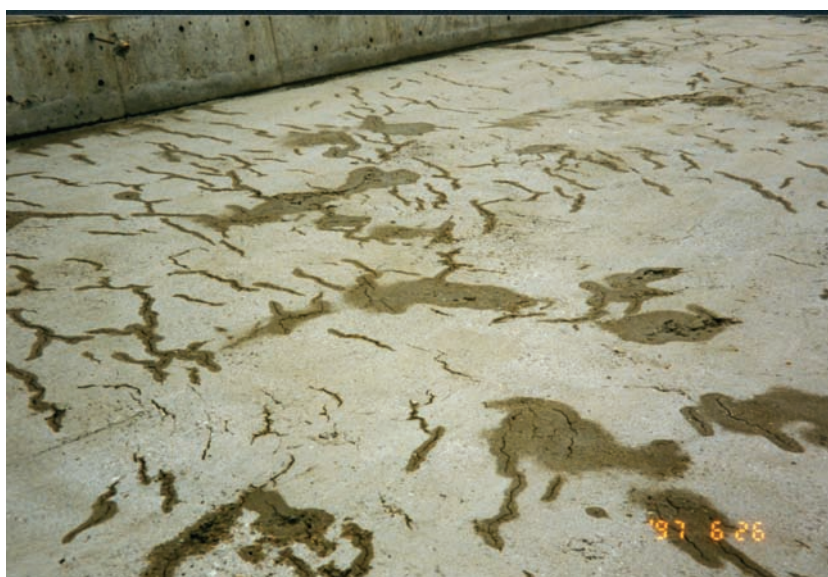
Fig. 3.2 Example of serious cracking due to plastic shrinkage (Photo: Reidar Kompen, Norwegian Public Roads Administration)
