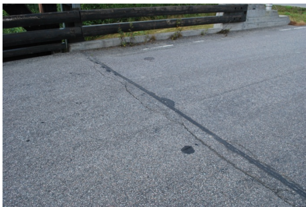
4-1516 Evenstad – sprekker i asfalten
