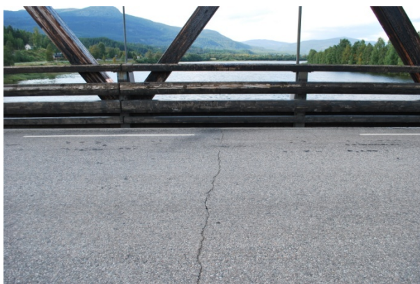
4-1516 Evenstad – sprekker i asfalten
