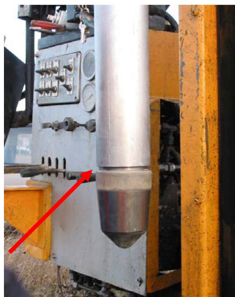
Figure 6 The cutting edge was not screwed completely
