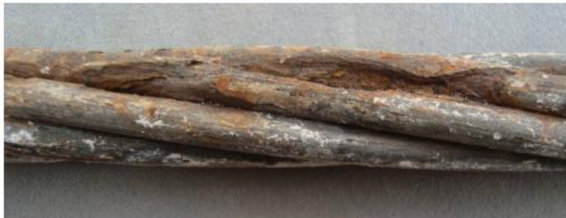
Figure 3: Example of corrosion attacks on a prestressing strand in contact with the whitish segregated grout [52]
