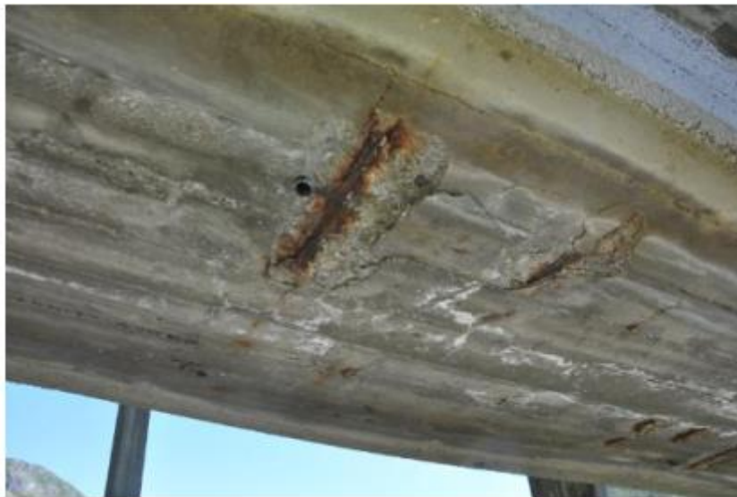
Figure 14: Reported corrosion at the arch elements
