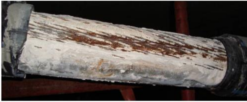
Figure 2: Example of whitish segregated grout embedding corroding strands [52]
