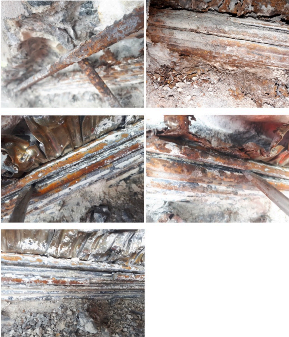
Figure E.2: Images taken from inspection site 2. Corresponds to image E1-5 to E1-9 in Appendix F, respectively
