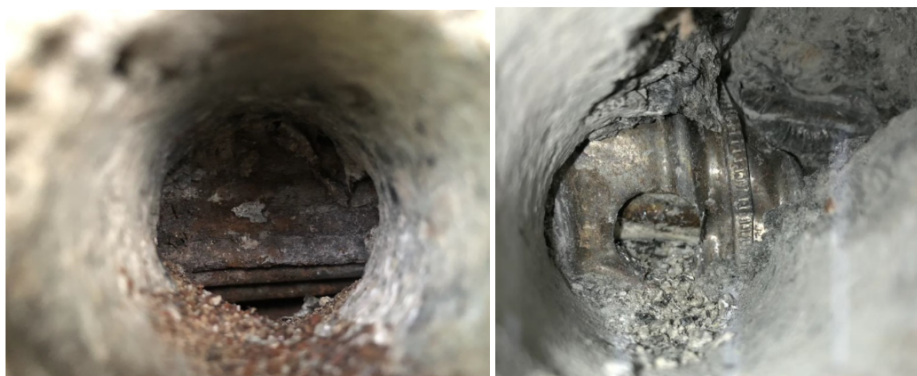
Figure 3.7: Tendon duct and tensile wires - Left: missing grout and corrosion on both duct and wires. Right: filled with grout and no sign of corrosion on either component [79].
