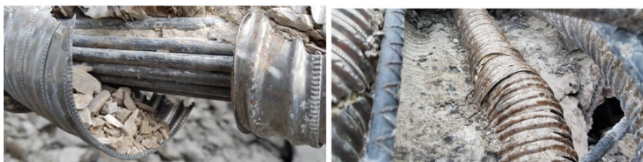
Figure 3.5: Images from Farriseidet bridge [79]. Left: tensile wires in a tendon duct covered in grout. Right: a tendon duct cast into the concrete.
