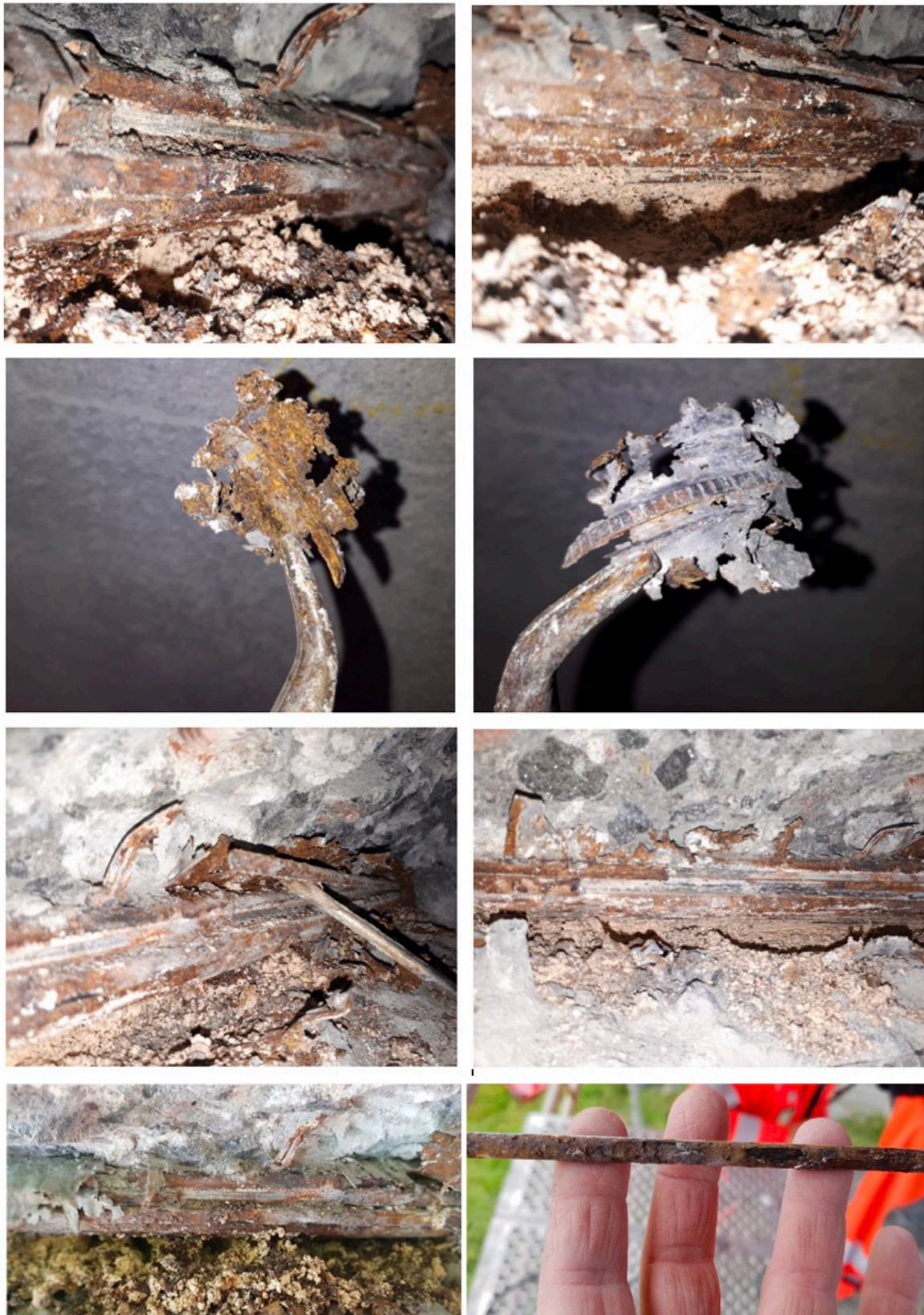
Figure E.3: Images taken from inspection site 3. Corresponds to image E1-10 to E1-17 in Appendix F, respectively
