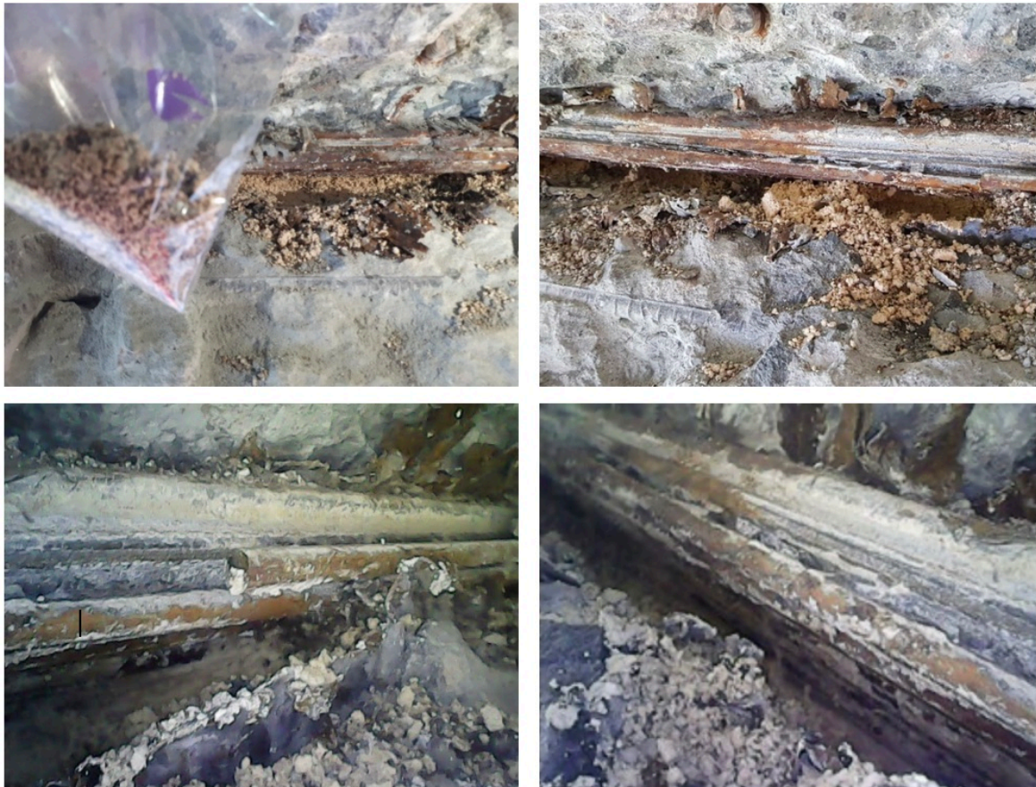
Figure E.6: Images taken from inspection site 3. Corresponds to image E2-8 to E2-11 in Appendix F, respectively
