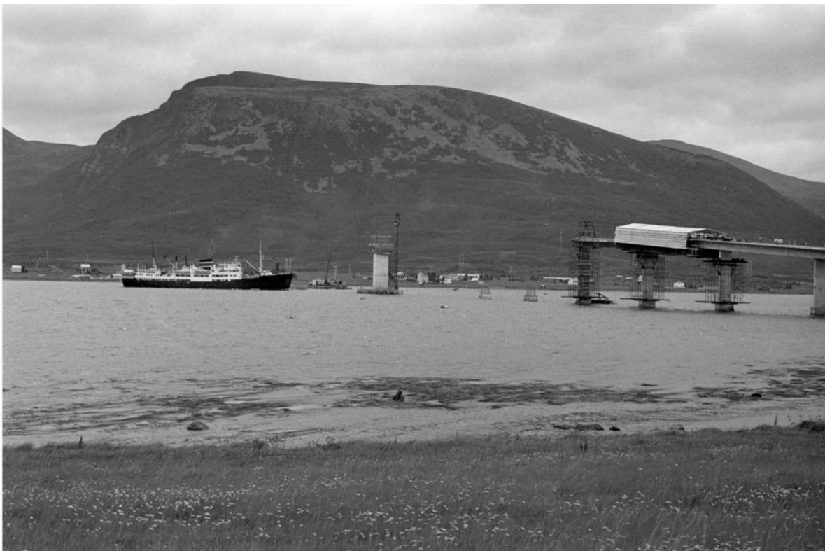
Figure 4-1 Picture of the building of Sortlandsbrua, picture taken from the north-western side of the bridge. Image from digitaltmuseum.no
