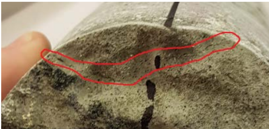
Figure 4-15 Core M6 with a crack
