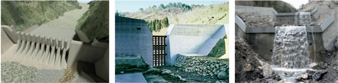
Figure 2.5: The left picture is a concrete slit dam in Madeira, Portugal (LCWConsult, 2015). The middle picture is a grid dam (nip) and the right picture is a series of closed check dams (Remaître et al., 2008).
