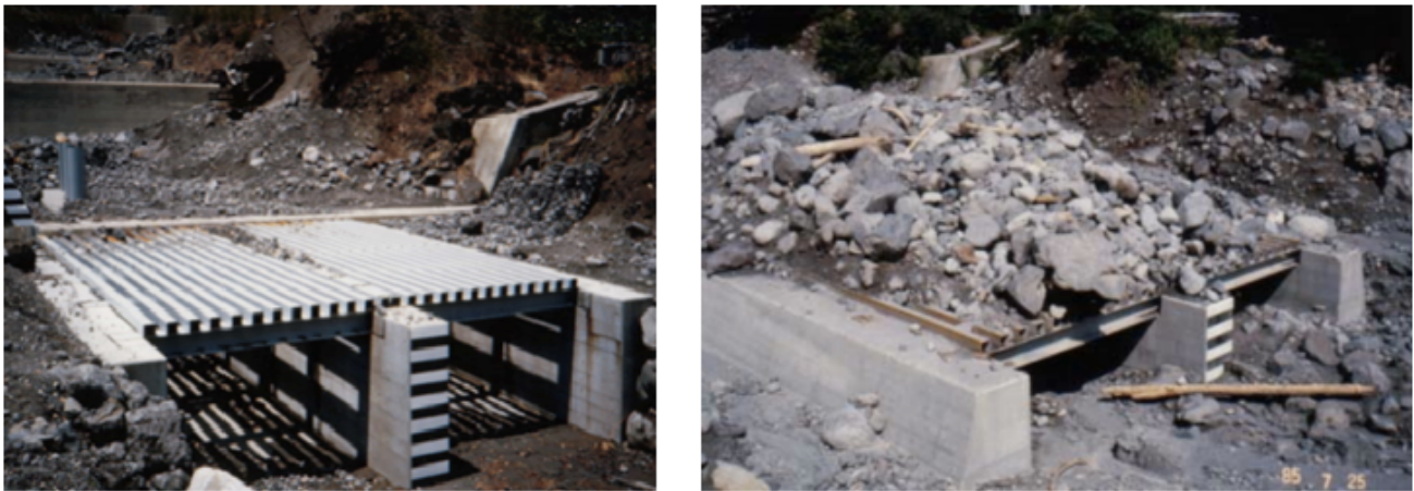
Figure 3.2: A 20 meter long and 10 meter wide debris flow breaker in Mount Yakedake, Japan. The left picture is before a debris flow has occurred while the picture on the right is after stopping the debris flow (Mizuyama, 2008)
