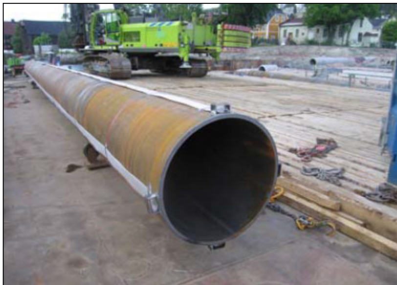
Figure 6. 4 The four vertical drains installed on the outside wall of the open ended steel pipe piles in axis 5 in the river. (30)
