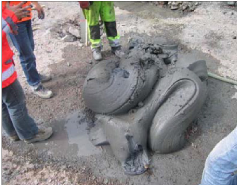
Figure 6. 5 The soft clay material (clay sausage) drilled/sucked out of the hole before driving the concrete pile. (30)
