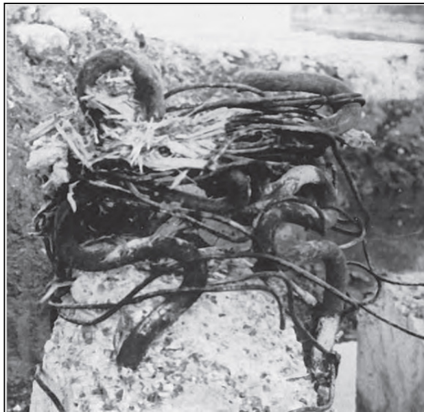
Figure 1. 5 Damage to head of precast concrete pile. (15)
