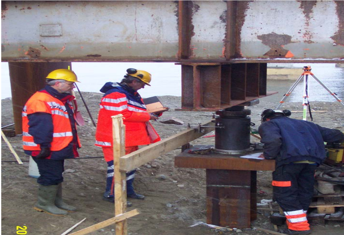
Figure 5.5 Typical pile load set up using adjacent piles in group for reaction (after Frode Oset)
