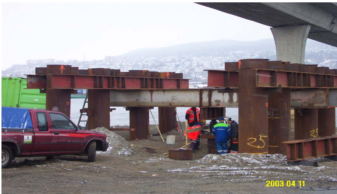
Figure 5.4 Typical pile load set up using adjacent piles in group for reaction (after Frode Oset)
