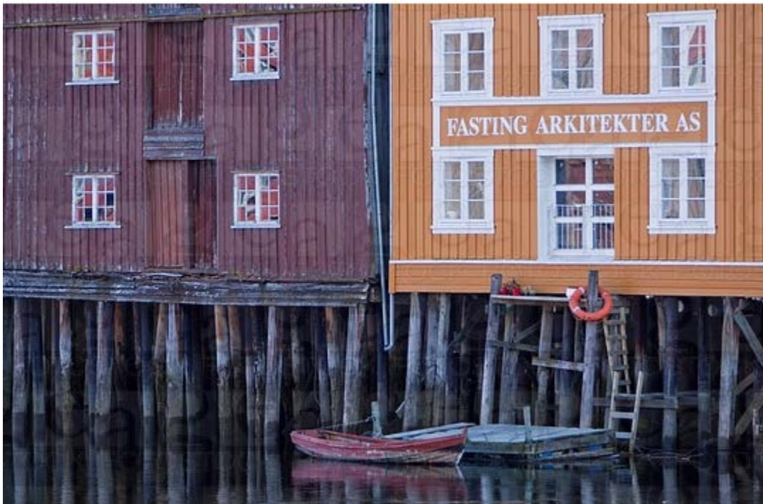
Figure 2.3 Timber piles used as foundation material in the city of Trondheim (after Ermias)
