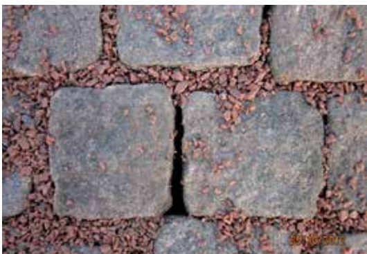
Figur V1.9 Mangelfull fuging (foto: René Kierstein)
