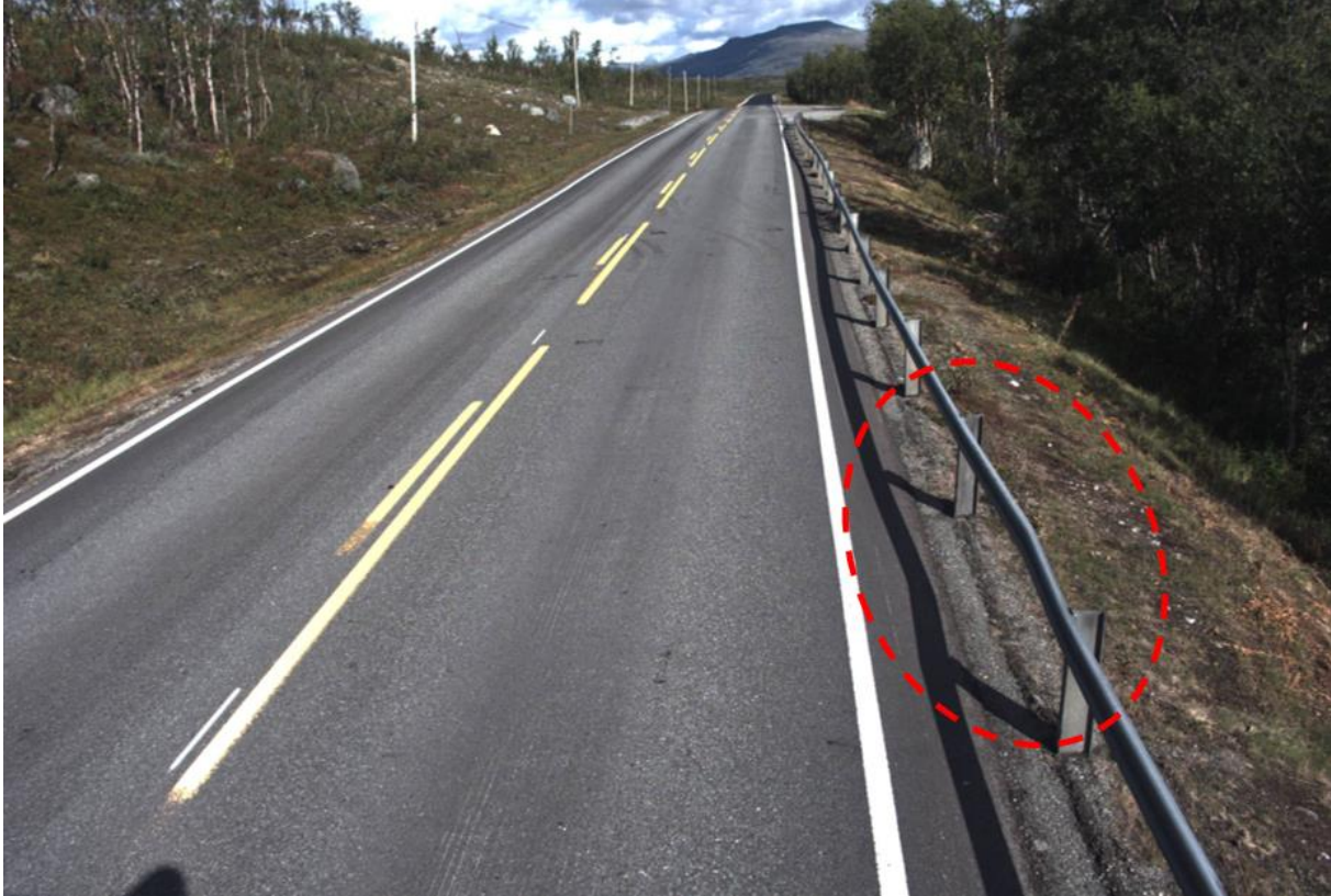
Figure 13: Example for a deformed guard rail.
