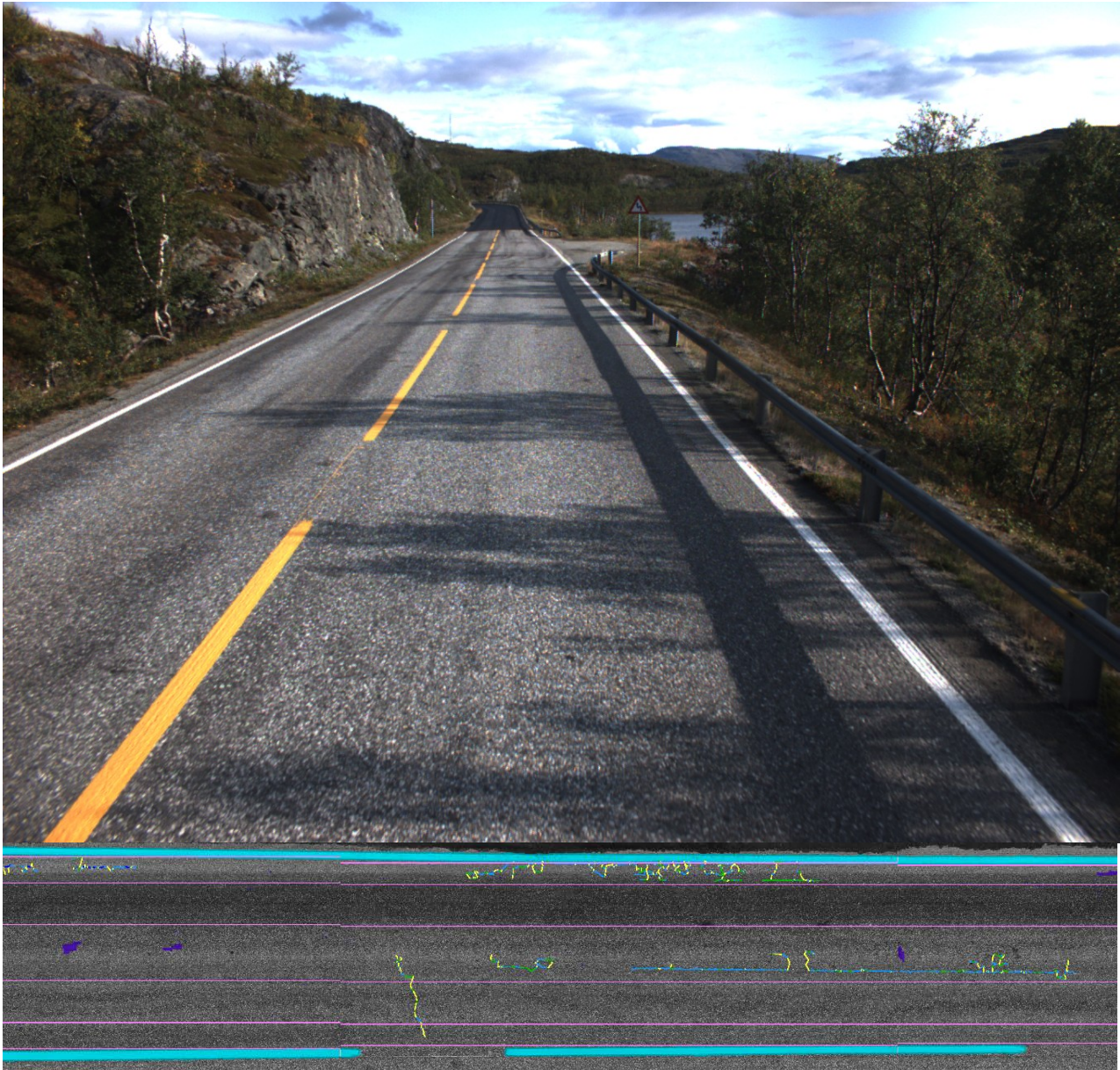
Figure 2. Front view image and LCMS overlay from direction 2, location 31 420
