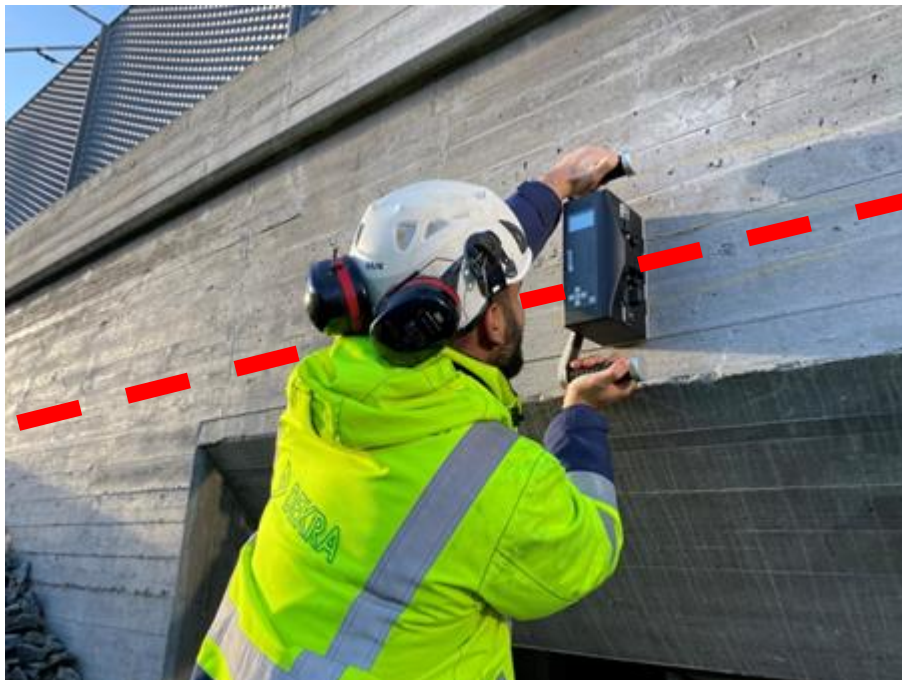
Fig. 8.8 Step 3 ; scans are carried out along the tendon duct with the instrument in a transverse direction relative to the tendon duct(s). Scanning requires a relatively smooth surface.
