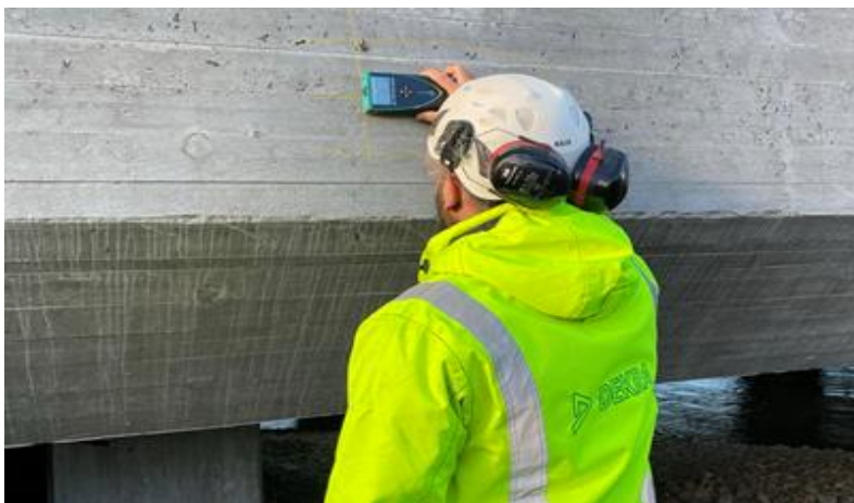
Fig.8.2 Step 1; Scan and mark out reinforcement in both x- and y-direction in the area intended for inspection.
