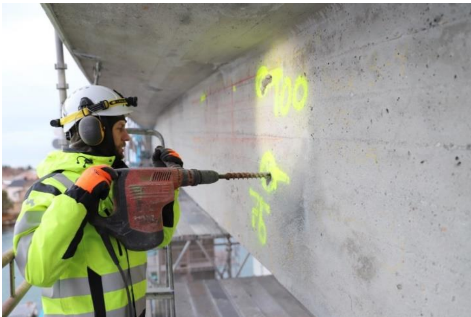
Fig. 8.16 Visual verification by drilling with a drill bit ( \text{\O}25 mm) into the duct wall.
