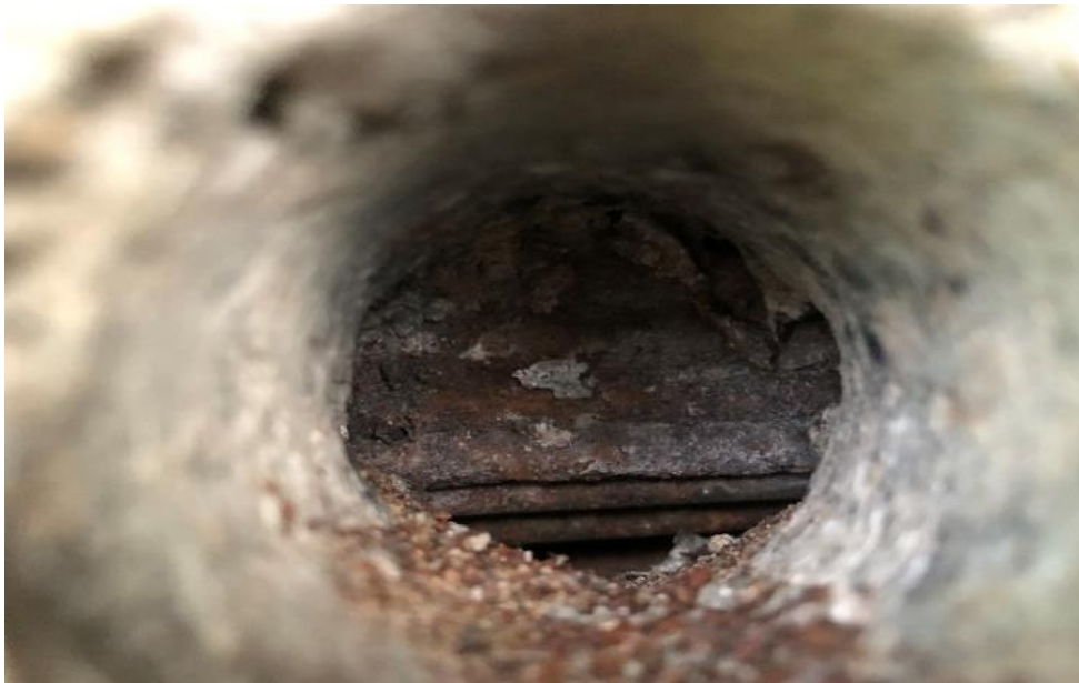
Fig. 8.17 Heavily corroded tendon after visual verification of air void by drilling with drill bit.
