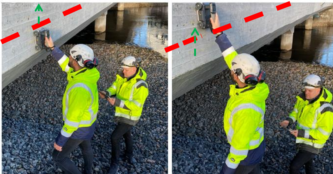
Fig. 8.5 Step 2; locating tendon ducts with GPR; scanning for localization is carried out in transverse direction relative to the tendon duct.
