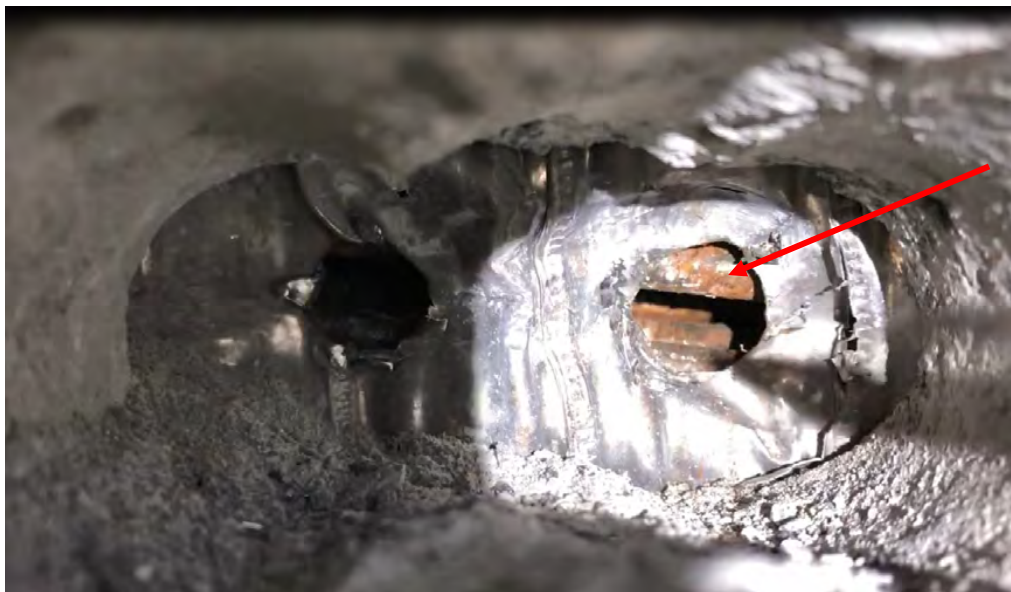
Photo no 6.1: Tendon duct 3SC with confirmed wire breakage
