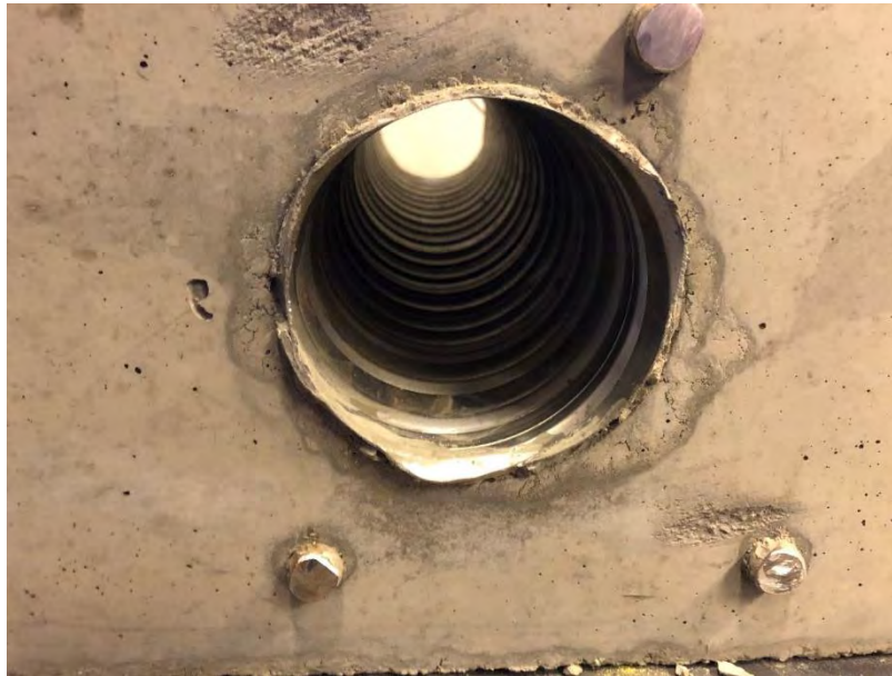
Picture 2.3 Empty duct B.
