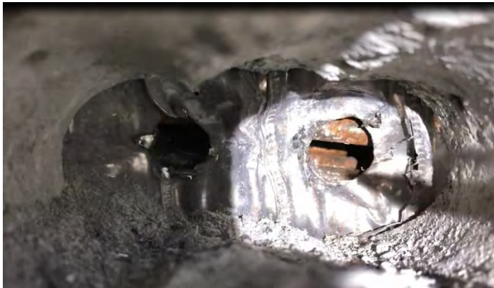
Figure 7.7 Visual inspection of tendons with missing grout
