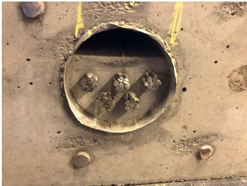
Picture 2.2 Duct A, Partially grouted (75%) half of the length and fully grouted the other half.
