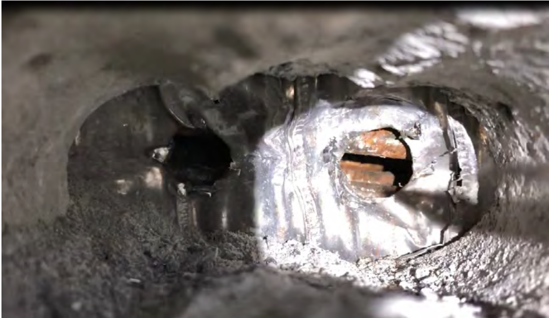
Photo no 6.4.3: Tendon duct 3SC with confirmed void and wire breakage
