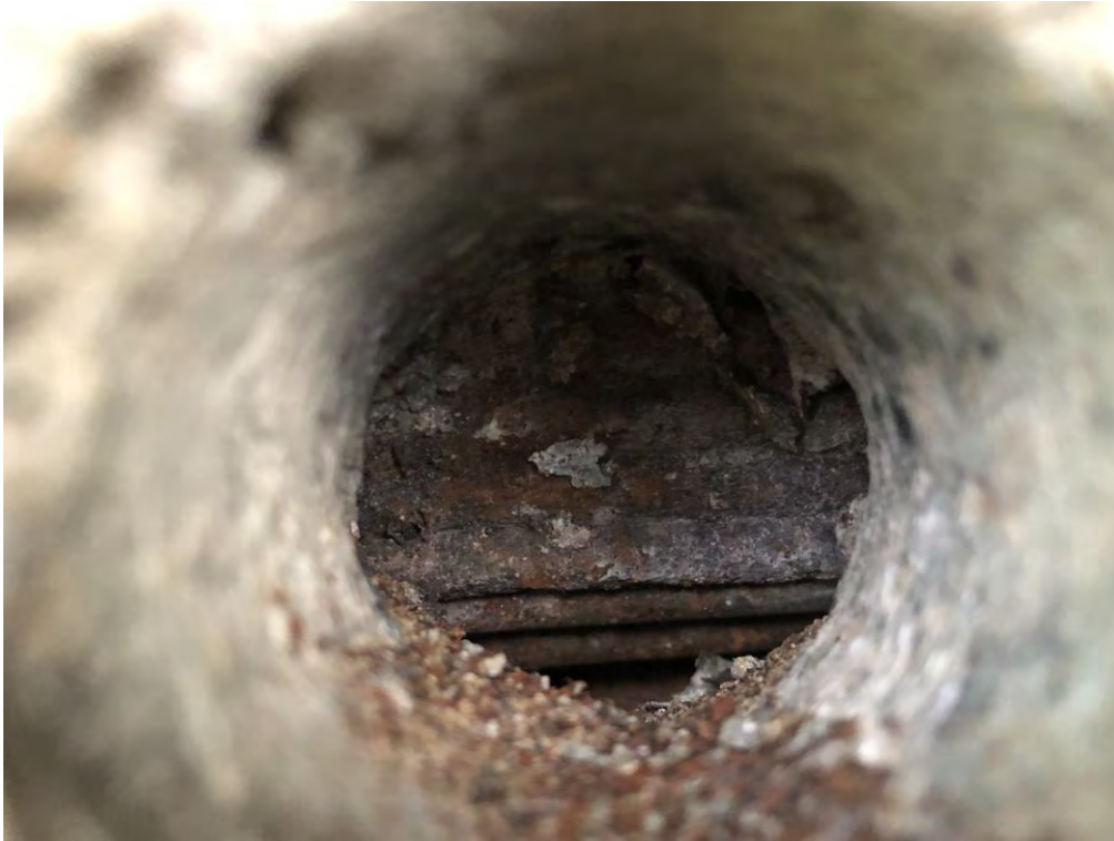
Photo no 6.3: Missing grout and corrosion in tendon duct 1NC.
