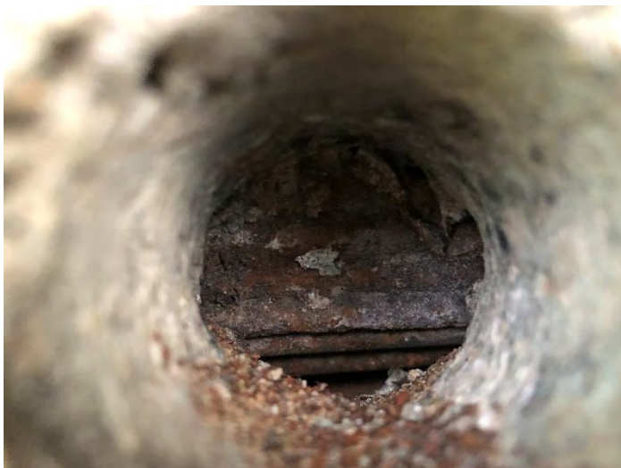
Figure 7.8 Missing grout and corrosion confirmed with visual inspection
