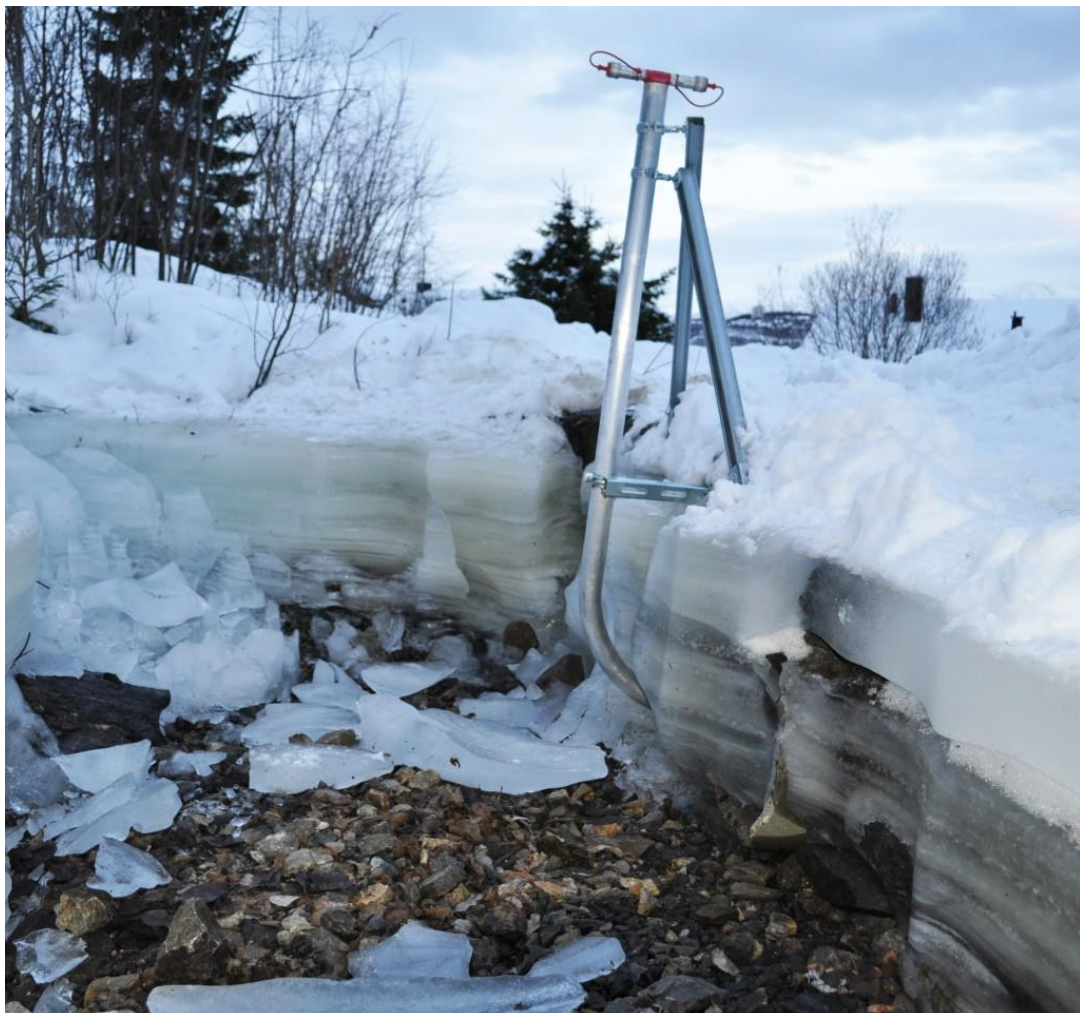
Ice Guard System – IGS, in-situ (Foto: Heatwork)
