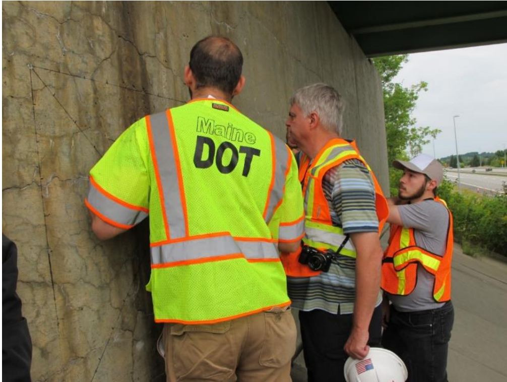
Figur 38 5th Parkway (Robertson Road) bridge over I-396. Site 6 (100 % silan). (Foto: Eva Rodum)
