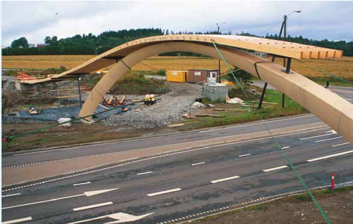
Figur 7-9: Tverrspent dekke med krumme limtrelameller. Leonardo da Vinci bru Figure 7-9: Stress laminated deck with curved glulam lamellas. Leonardo da Vinci Bridge
