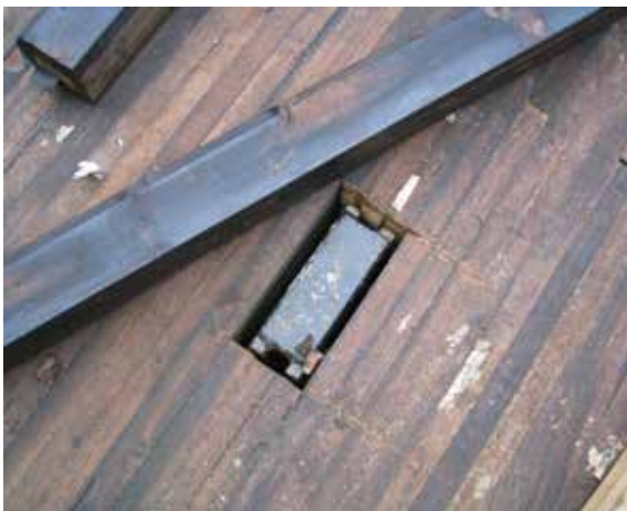
Figur 7-13: Innfelt sidestyling i dekket før utstøpping, Ner-Hole bru Figure 7-13: Recessed lateral support in the deck before grouting, Ner-Hole Bridge
