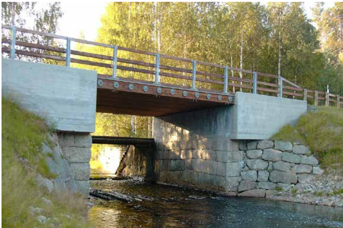
Figur 6-6: Mattisdammen bru (2000) har en tverrspent plate av limtrebjelker. Spennvidde 7,2 m Figure 6-6: Mattisdammen Bridge (2000) has a stress-laminated slab made up of glulam beams. Span 7,2 m
