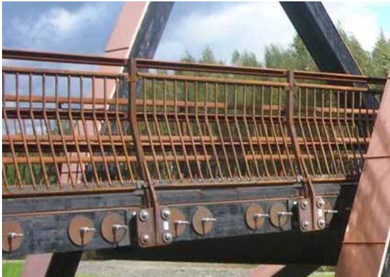
Figur 7-25: Kjøresterkt rekkverk med grind. Utførelse i rusttregt stål. Figure 7-25: Vehicle restraint barrier with grillage Make in weathering steel.
