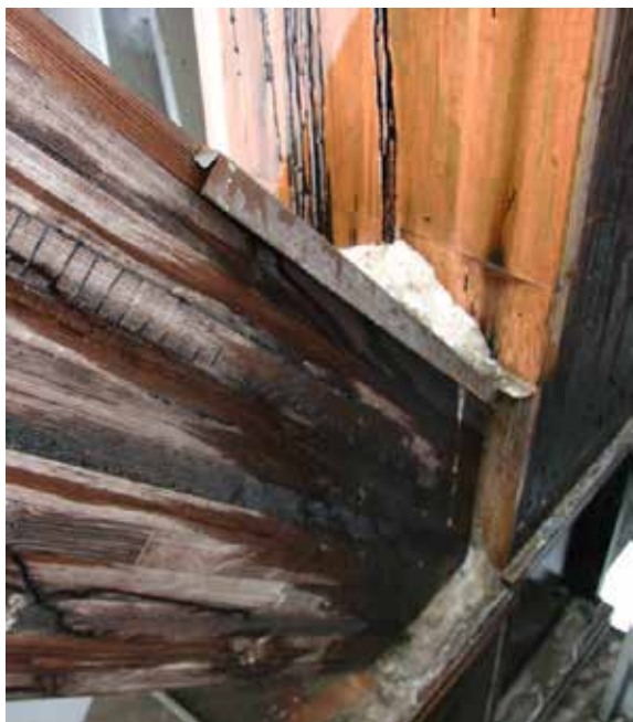
Figur 10-12: Kobbertekking avsluttet i en sliss. Figure 10-12: Copper cladding terminated in a slot.
