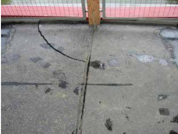
Figur 10-15: Sprekker i støpeasfalt Figure 10-15: Cracks in mastic asphalt surfacing
