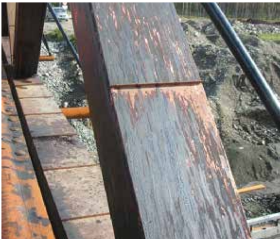
Figur 7-26: Sterk kreosotsvetting fra fagverkets overgurt. Figure 7-26: Excessive creosote bleeding of the truss' upper chord.
