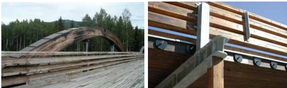
Figur 7-22: Kjøresterkt rekkverk for blandet trafikk – Daleråsen bru Figure 7-22: Vehicle parapet for mixed traffic – Daleråsen Bridge
