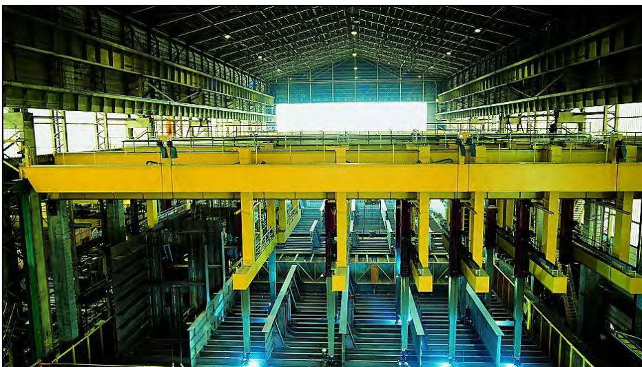
Figure 16-5 Large robotic welding station at OSS Lindø shipyard
