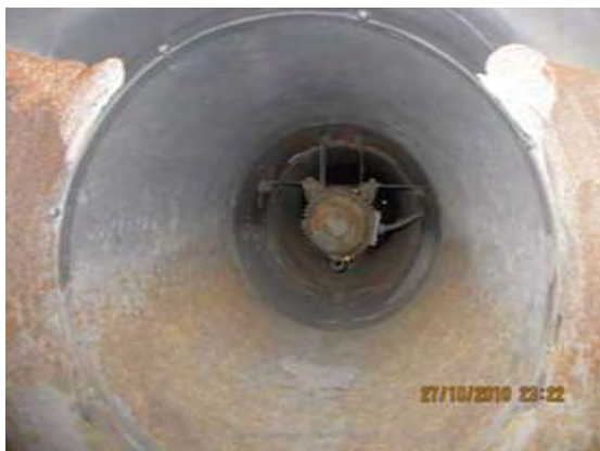
Figur 8. Old ventilator after corrosion.
