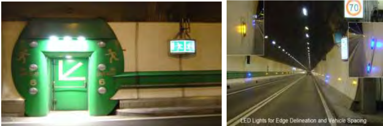
Figure 14 and 15: Examples of escape route, signs and LED lights used in modern road tunnels.
