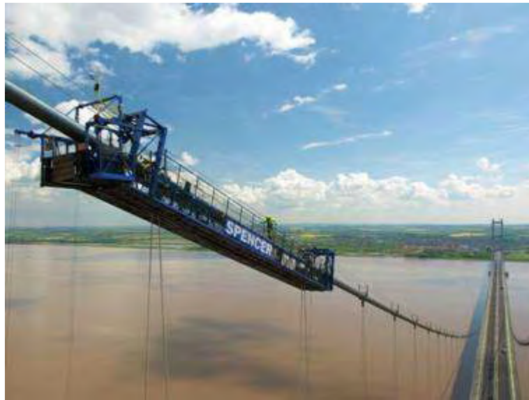
Figure 2 - Spencer Cable Crawler, Installed At Humber Bridge, UK
