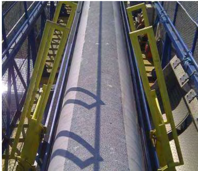
Figure 7 – Neoprene Wrapped And Anti Skid Painted Cable
