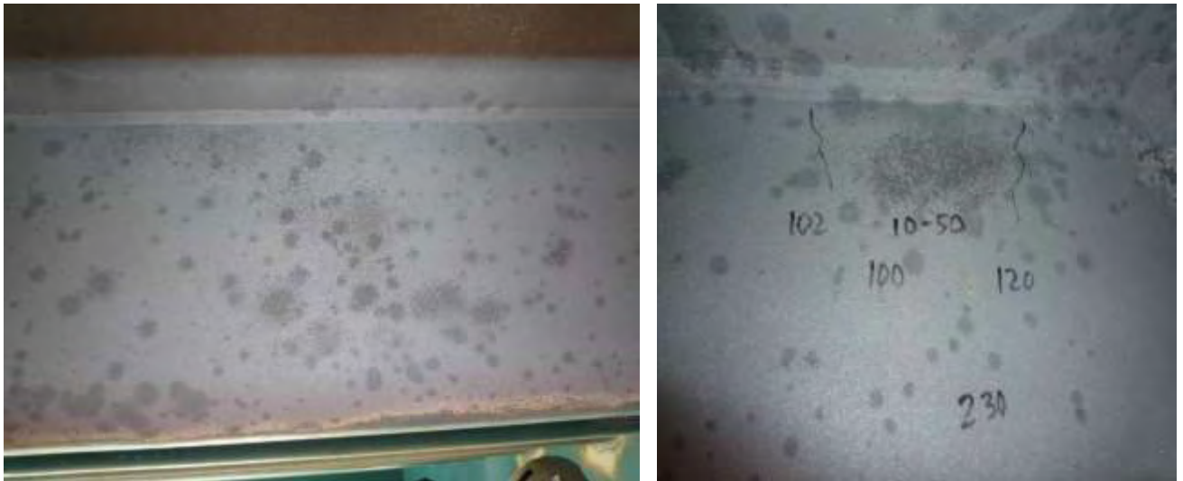
Photo no. 9 Removal of coating system down to zinc coating. The dark, spotted areas have a DFT lower than the light grey areas due to corrosion after 22 yrs of service on the Bergsøysund Bridge
