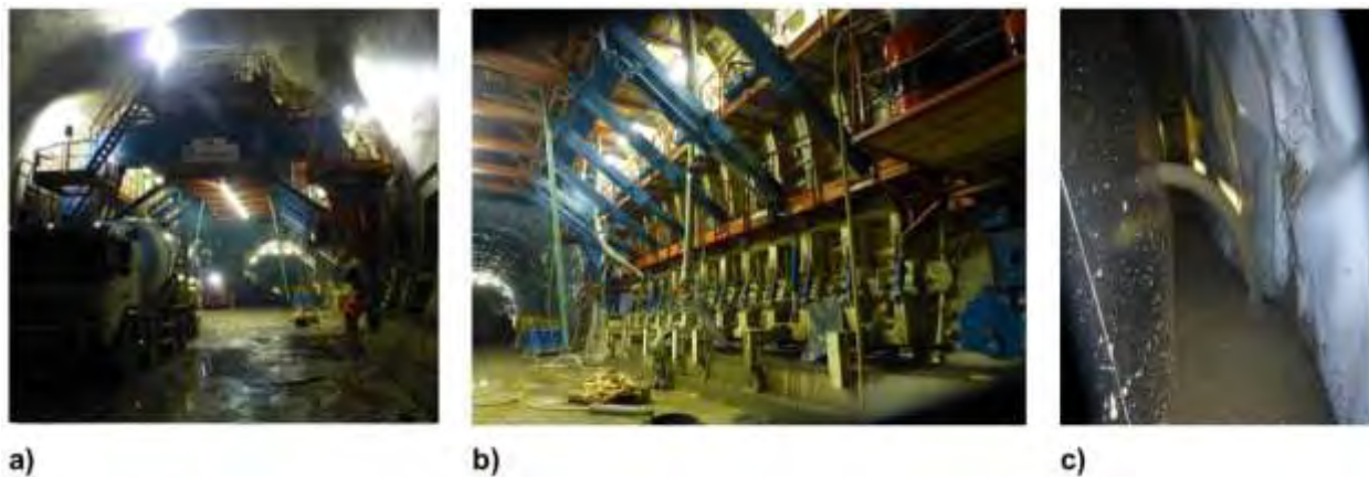
Figure 12. (a) Formwork; (b) steel structure of the formwork; (c) concreting (left: formwork, right; sealing membrane).
