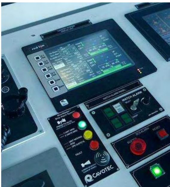
Figure 39: Typical Ferry Bridge Installed Equipment
