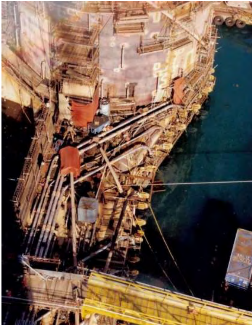
Fig. 6. Piping routed on pontoon top.
