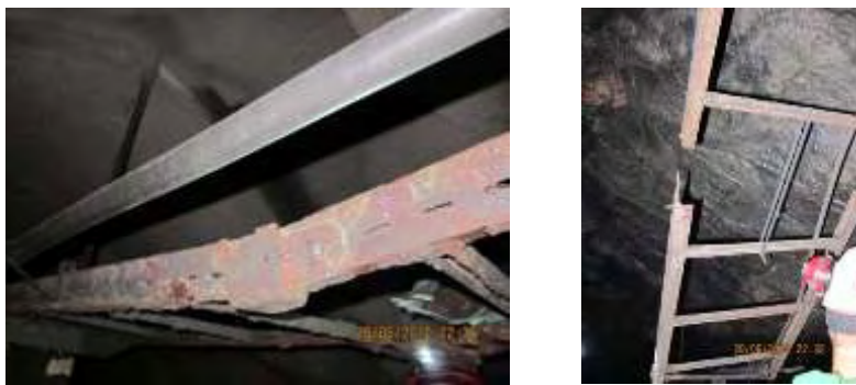
Figur 10. and 11. Examples of broken cable bridges due to corrosion in Norwegian tunnels.
