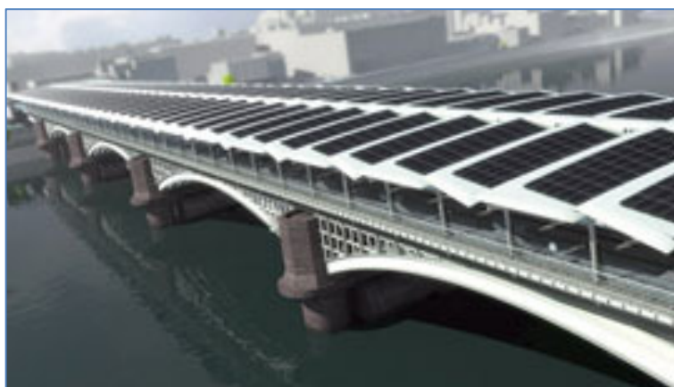
Blackfriars Bridge (London, UK). Railway bridge. Currently under construction. 4 400 panels are being installed (Solarcentury)
