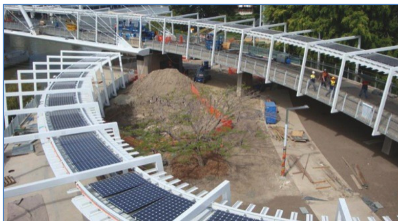
Kurilpa Bridge (Brisbane, Australia). Walkway bridge completed 2009. 84 panels installed (Sunpower)
