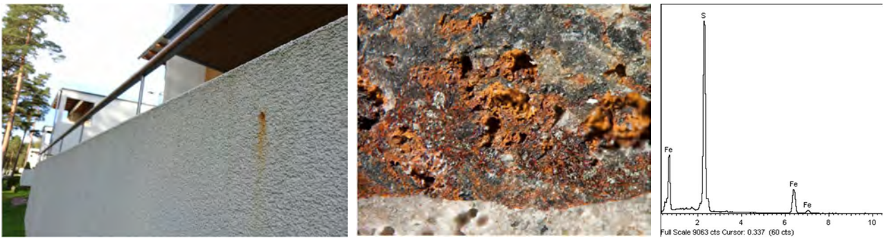
Fig. 1. Damages caused by sulphide minerals on the surface of a concrete panel.
