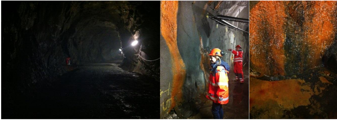
Figure 1. Photos from left to right: the tunnel at the test site, one of the tunnel locations with extensive biofilm formation and close up of the biofilm on the sprayed concrete.
