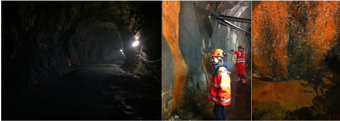
Figure 1. Photos from left to right: the tunnel at the test site, one of the tunnel locations with extensive biofilm formation and close up of the biofilm on the sprayed concrete.
