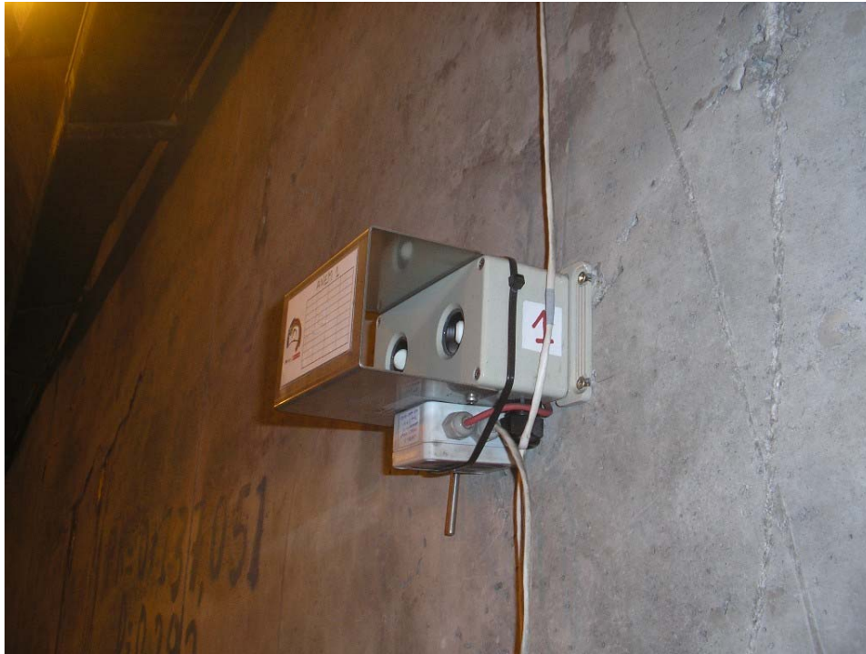
Photography 4.1.1.VI. – Anemometer installed in the Bielsa Tunnel.
