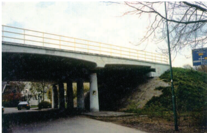
Fig. 7.1. First structure in which ASR was recognized in the Netherlands, Schoonhoven bridge (Picture W. Heijnen, 1991).
