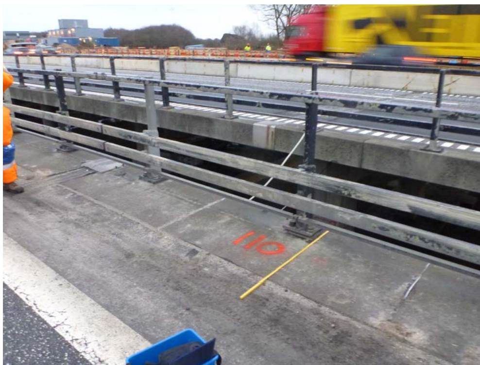
Figure 14 - Karlstrup Mose highway bridge. Edge beams containing varying amounts of fly ash. Photo courtesy Kirsten Eriksen
