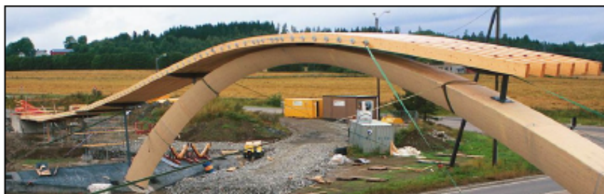
Figur 7-9: Tverrspent dekke med krumme limtre lameller. Leonardo da Vinci bru Figure 7-9: Stress laminated deck with curved glulam lamellas. Leonardo da Vinci Bridge
