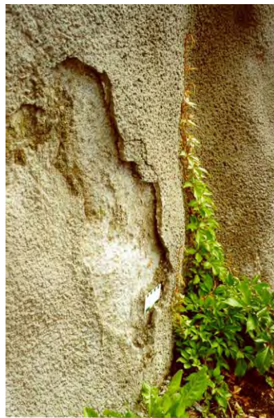
Figure 1. Spalling in steel fibre reinforced sprayed concrete due to thaumasite sulfate attack and associated carbonation (Hagelia and Grønhaug 2000).
