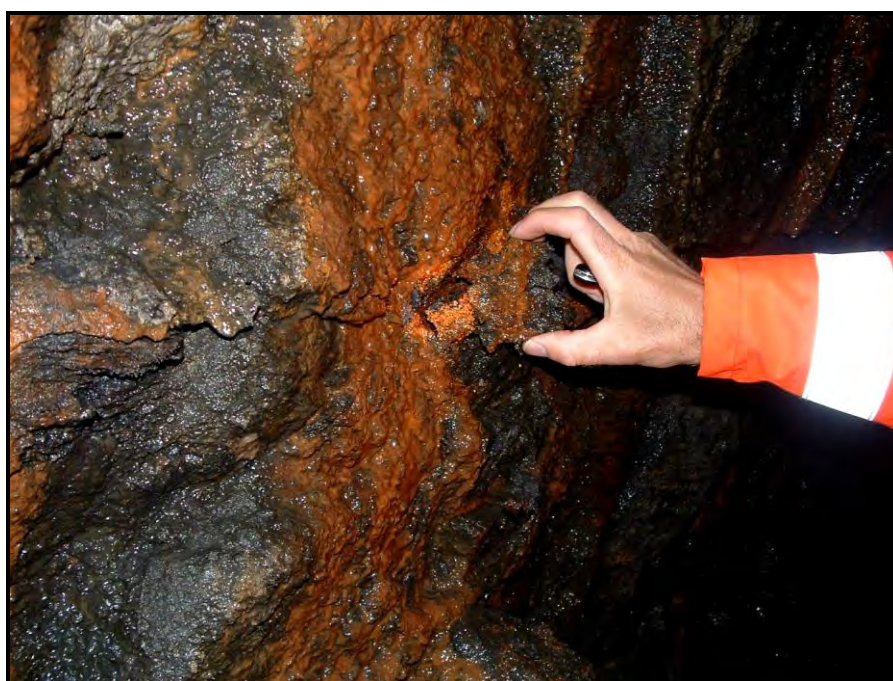
Figure A5-4-8: Freifjord subsea tunnel. Extensively deteriorated sprayed concrete due to interaction with Mn-Fe biofilms and saline ground water. pH = 5.8 in small leakages. Black and rusty crust material consisted of Na-buserite (hydrous Mn-oxide biomineral), amorphous Fe (likely ferrihydrite), the clay minerals vermiculite and dickite (with a \text{HCONH}_2 group), quartz and plagioclase. Situation from June 2006: concrete age 16 years.
