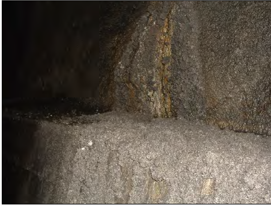
Figure A5-4-13: Freifjord subsea tunnel. Concrete age: \approx 16 years. Very extensive deposition of gypsum mush associated with a leaky crack through weathered decalcified, friable and rust stained sprayed concrete, running over a cast concrete banquette (“Rivers of gypsum”). On either side the sprayed concrete was covered by a similar thin gypsum deposit.
