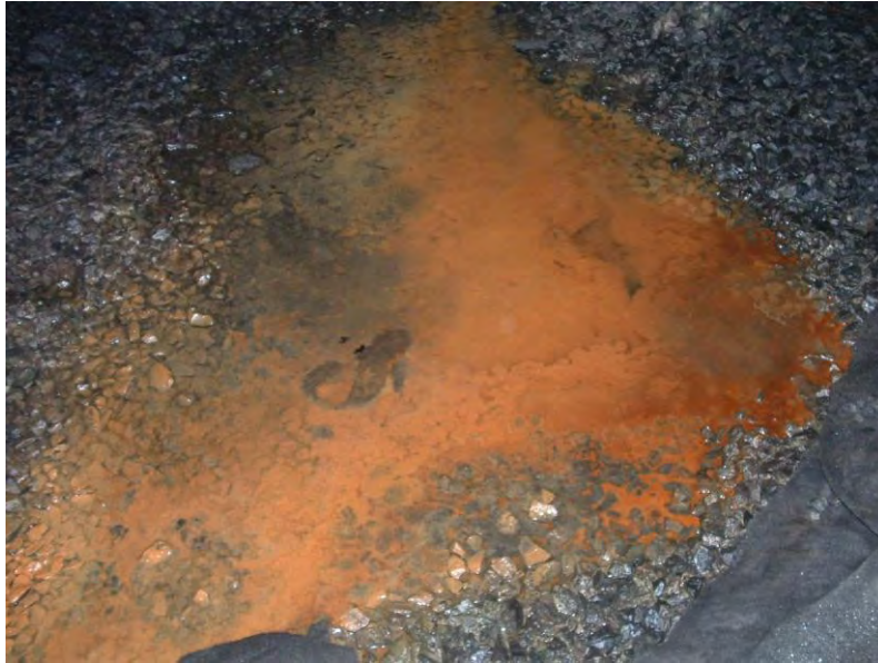
Figure A4-5-1: Svartdal tunnel water sample 320-06 and rusty and dark bacterial slime was collected from this pond just beneath the Alum Shale core sample station (before drilling).
