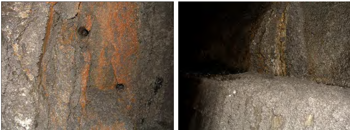
Figure 5: Freiffjord subsea tunnel at concrete age 16 years. Left : Extensive breakdown of sprayed concrete attacked by saline ground water and Mn-Fe biofilms, overlain by grey carbon bearing gypsum mush. Notice the partly erased old core holes: Image width = 140 cm. Right : Thick carbon bearing gypsum deposit on cast concrete banquette derived from a leaky crack through decalcified and friable sprayed concrete. Image width = 200 cm.
