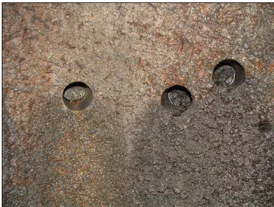
Figure A5-4-11: Freifjord subsea tunnel in 2006. Concrete age: \approx 16 years. Surface deposits of gypsum with some crystalline carbon precipitating from saline water draining at the concrete/rock interface. Core 6150-2 from 2003 = left hole with pH = 6.2 in 2006. The other cores were older and had accumulated much more gypsum. Note the smoothed rust stained and bleached concrete surface. Gypsum formation consumes acid suggesting pH in water behind the sprayed concrete layer was < 6. The carbon was derived from dead bacteria occurring at the concrete/rock interface. Core holes ( \Phi = 50 mm).
