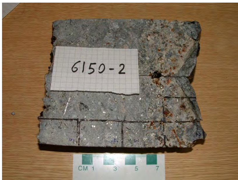
Figure A5-4-14: Freifjord subsea tunnel. Concrete age: \approx 13 years. Core 6150-2 with 45-50 mm degraded friable sprayed concrete and destructive steel fibre corrosion within Layer A against the rock mass (right). The degradation was characterised by Mg ingress (forming MCSH and brucite) and local Thaumassite Sulfate attack (TSA) at the transition to more sound concrete. Calcite, laumontite, aragonite and nordstrandite also occurred. Impact from microbial activity acting from behind the spray was indicated by the presence of several phosphate minerals, a possible phenyl phosphate hydrate (Table A-5-2) and a carboxylate (an organic mineral) formed: a) within concrete 3 mm from the concrete/rock (Figure A5-4-15) and b) as a microscopic thin deposit on the outer surface (left).
