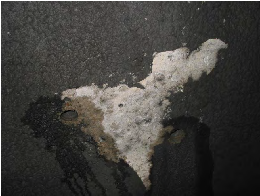
Figure A6-3-1 Spalling in dry extensively carbonated sprayed concrete at chainage 43720 m in the Lier tunnel. Two 50 mm cores were extracted for thin sectioning. The concrete was frequently sounder deeper inside, yet showing evidence of a sulfate attack in previous years. The dark outer surface represents dusts mainly consisting of carbon and iron.
