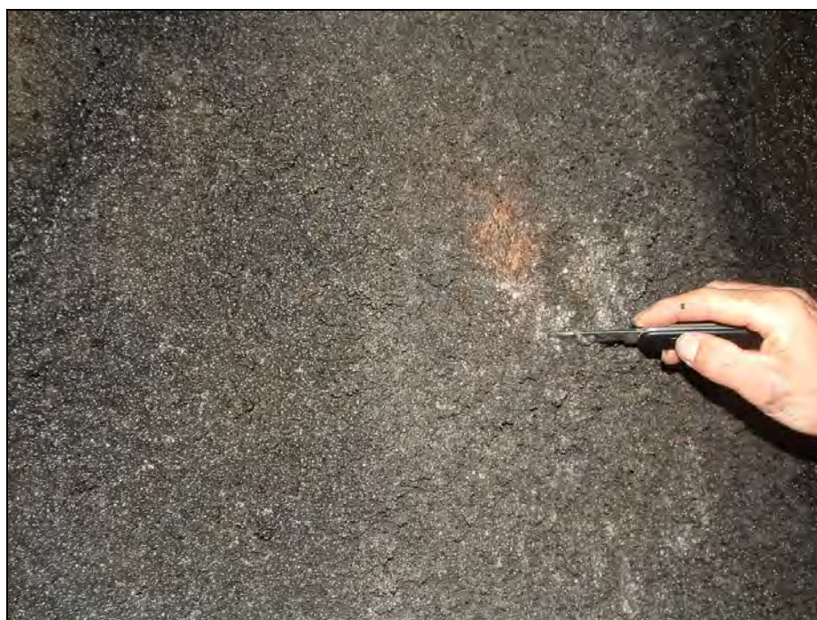
Figure A5-4-12: Freifjord subsea tunnel. Concrete age: \approx 16 years. Gypsum deposit with crystalline carbon (5-10 mm thick).
