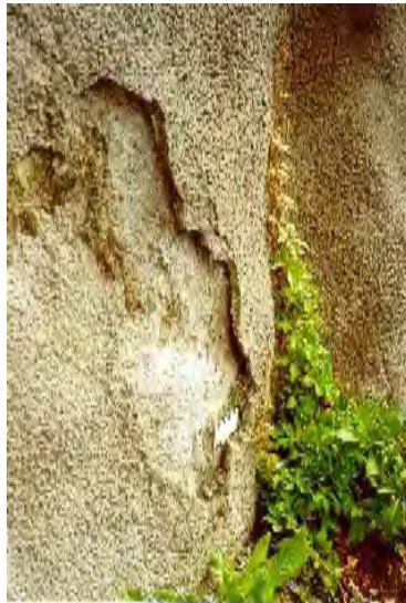
Figure 4: Spalling after less than 13 years in a 1987 steel fibre reinforced concrete (SRPC and SF), due to TSA and carbonation due to PCD. A previous spray had been severely affected and was replaced after 17 years in service. Alum Shale environment, Åkebergveien Oslo.
