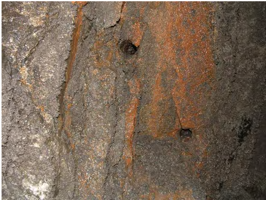
Figure 6: Old core locations in the Freifjord subsea tunnel showing extensive breakdown of the sprayed concrete 16 years later. Rusty and black areas (right) consist of iron oxihydroxide from Gallionella ferruginea and manganese oxides derived from Leptothrix sp. Grey deposits consist of gypsum formed from Ca in concrete and sulfate from seawater.
