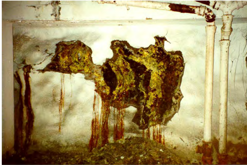
Figure A1-4-1: Effects of swelling Alum Shale and sulfate attack in abandoned civil defence shelter in 2000. This now ca. 40 years old (in 2010) sprayed concrete was made with SRPC (dry method, no steel fibre reinforcement). The thickness was about 5-6 cm and severely infected by TF-TSA-carbonation associated with ettringite and gypsum. The cement paste matrix was severely leached and porous. The exposed Alum Shale surface was heavily coated with secondary jarosite and also carried gypsum and iron-oxyhydroxides. Notice the heavy accumulation of completely disintegrated concrete fragments at the base. Image width = 3 m.
