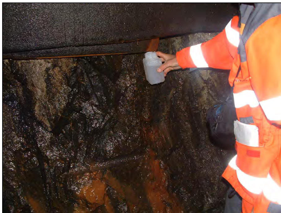
Figure A5-4-9: Freifjord subsea tunnel. Sampling of water 4930-1 from leakages draining across a water panel within 15-20 meters of the location in Figure A5-4-8. The water leakages behind this panel were associated with Mn-Fe biofilms, showing extensive interaction with degraded concrete in the tunnel crown. The water was brackish (Table 2, Chapter 7) and sulfur isotopes showed very significant influence of sulfate reduction (Table 9).
