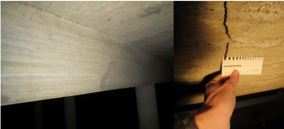
Figure 4.7: Cracks appearing at the original zero moment section (eastern inner beam) between axis 6-7, 4,5m before axis 7. (Aas Jacobsen, 2013)
