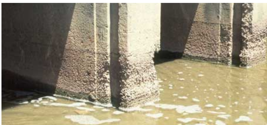
Figure 2.3: External sulfate attack
