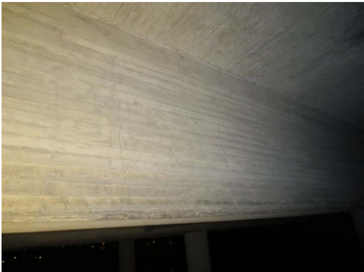
Figure 4.8: Typical cracks occurring in the field sections. Closed in bottom and top. (Picutre taken between axis 5-6) (Aas Jacobsen, 2013)
