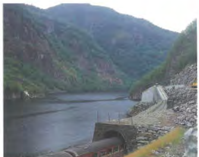
Road under construction at Dale near Voss in Hordaland. Photo: Erling Grønsdal
