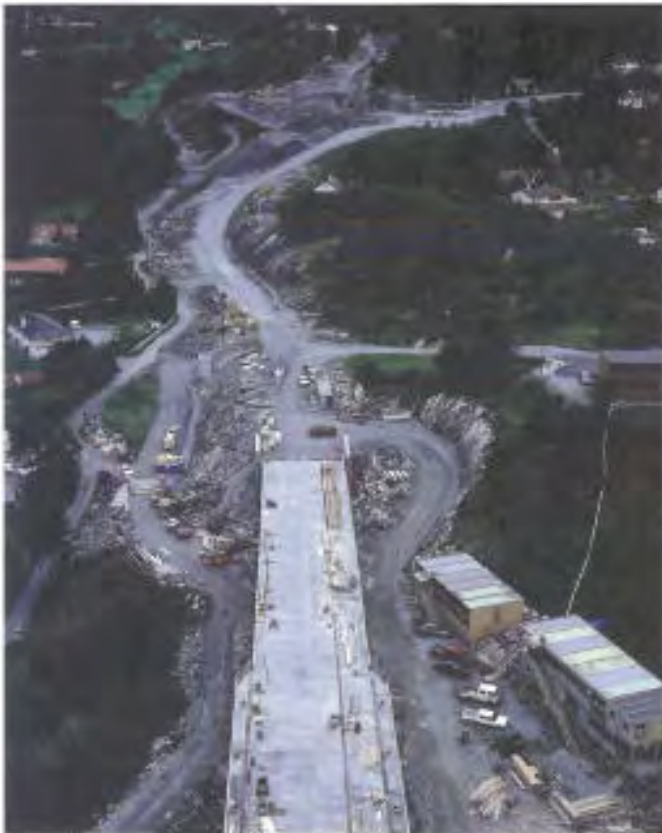
Site where equipment and stores are kept, Salhus bridge in Hordaland. Photo: Erling Grønsdal
