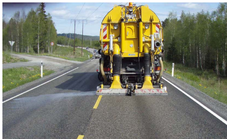
Figure 4 Cleaning of porous asphalt pavement on Highway 170, equipment from the Oslo Airport Authority, Gardermoen
