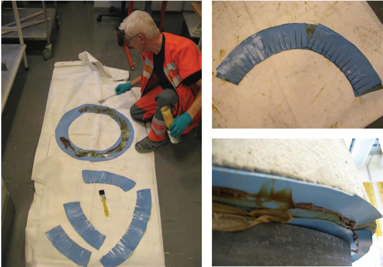
Fig. 5.4 Two layers of PVC-membranes and grease as bedding material. Preparation of grease on the bottom membrane layer (left), the cut membrane is placed on top (top right) and slide freely during testing (bottom right).
