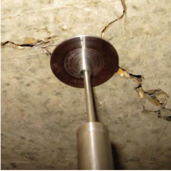
Fig. 5.2 Measurement of central displacement at the bottom side of the panel by the use of a spring loaded displacement transducer (LVDT) with a disc on top which can rotate along with the rotation of the panel, as well as bridging over the cracks.
