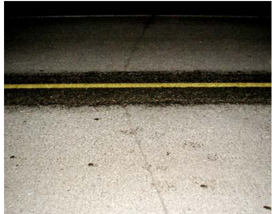
Figure 4: Inclined joints after approximately 15 years service. Longitudinal centre joint was repaired after uncontrolled cracking.
