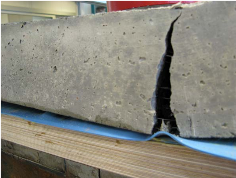
Fig. 6.8 Example, “no friction” conditions: Lifting of panel edge, opening of a crack and sliding (in the grease layer) along the inner edge (not visible) of the support. Sliding takes place between the cut upper plastic sheet layer (blue) and the plastic layer below (grey).
