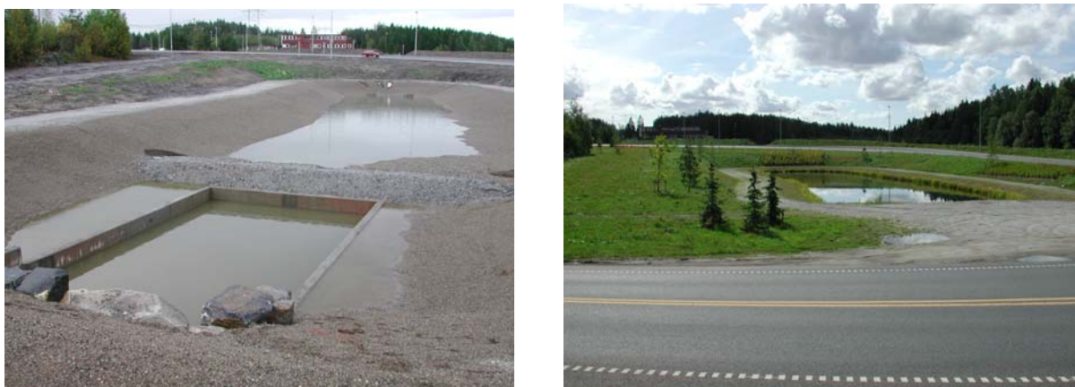
Figure 10: Stormwater pond for treatment of surface water E6 at Taraldrud in Ski municipality Norway) with integral soakaway and water depth in the main pool of 2.5 m (Photo: Roger Roseth).
