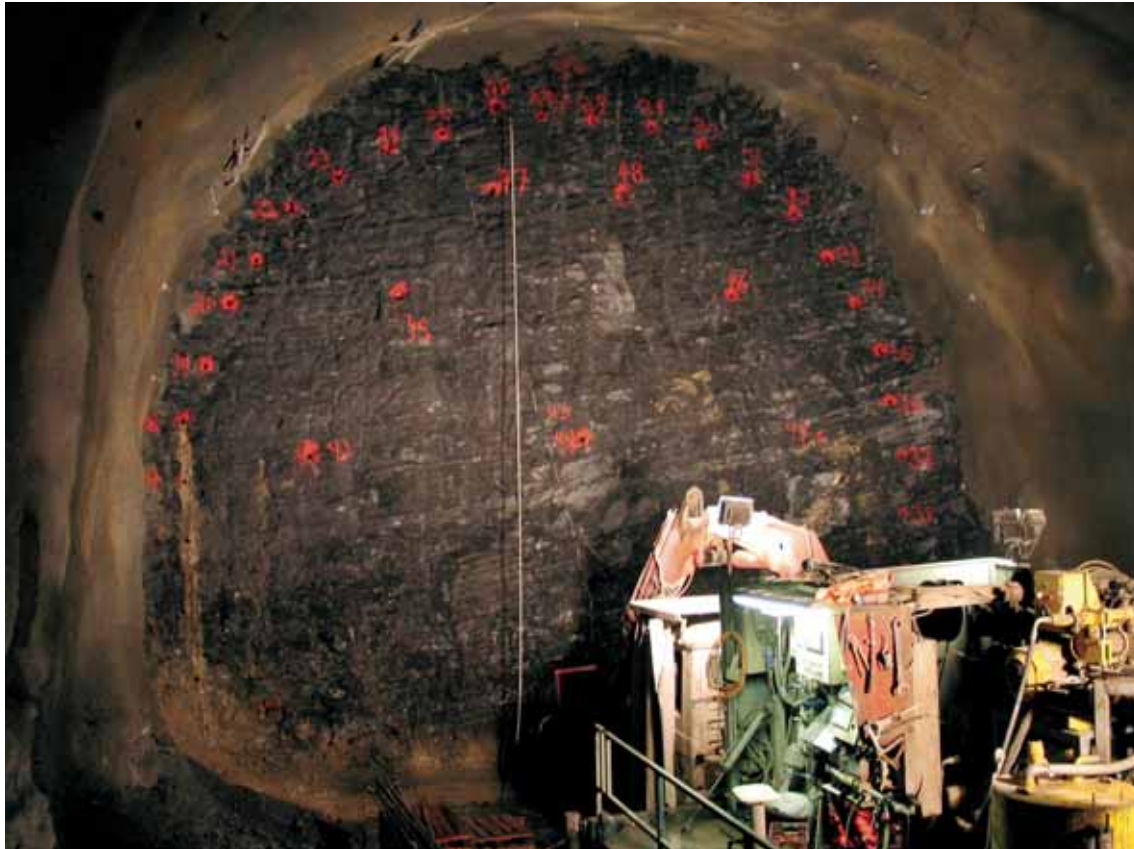
Figure 15 The Tanum tunnel (Jong-Asker railway). Markings of injection holes in the tunnel work face.
