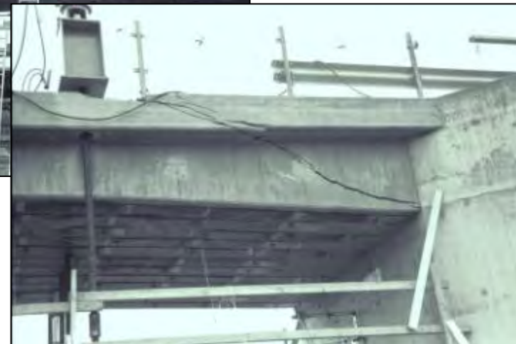
Shear failure at ca 460 ton
