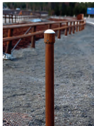
Fig. 4. The road lighting installation with LED
