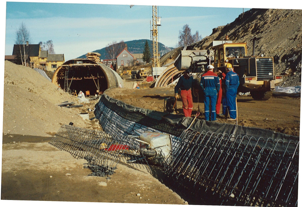
Fig. 2 Steel mesh in the front with vegetation mat. Construction of the third lift
