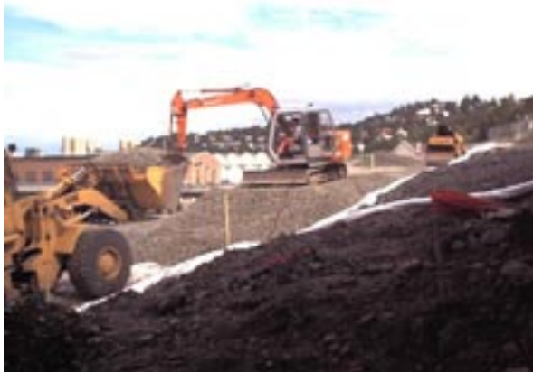
Figure 5: Distributing foamglass material using a crawler mounted excavator (Hitachi EX60, 8 tonnes). For internal transport on site a shovel dozer (CAT 923E) was used.
