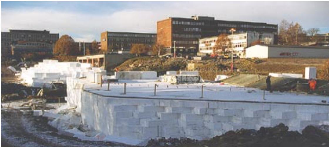
Figure 1: An EPS embankment with vertical walls for a city tramline in Oslo as an alternative to a bridge.
