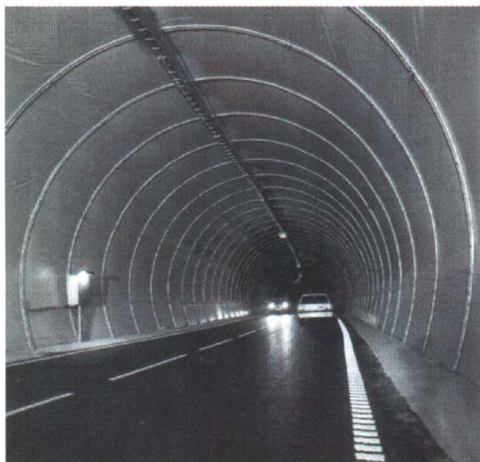
Figure 6: Lining made by PVC/polyester tunnel fabric.
