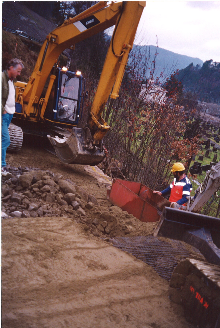
Fig. 4 Moving the formwork with the machine. Sandy gravel used as backfilling material, compacted to minimum 97 % Standard Proctor
