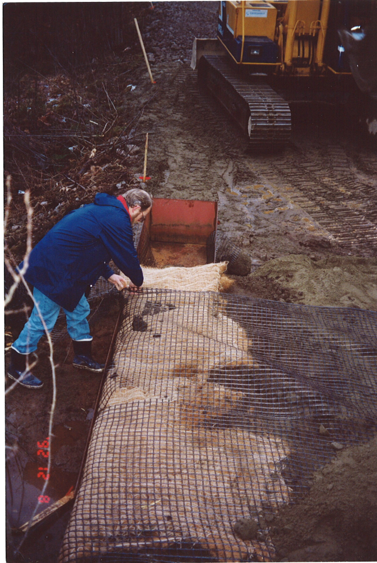
Fig. 3 Steel box used as formwork in the front. Telegrid 55/30 with spacing 0,5 m used as reinforcement. Vegetation mat used in the front to speed the vegetation process
