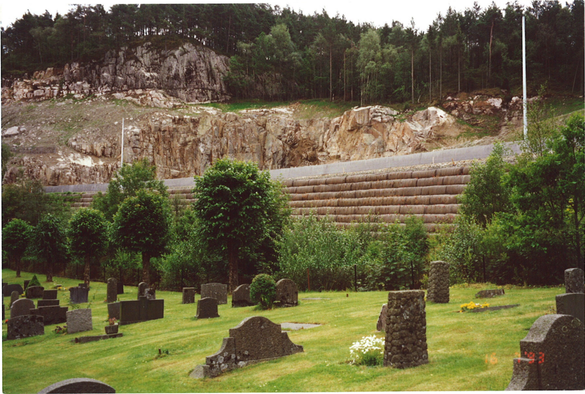
Fig. 6 Finished reinforced 60 ° slope with maximum height 7,0 m and reinforcement length 5,0 m. Total cost 580 NOK/m 2 (83 $/m 2 )
