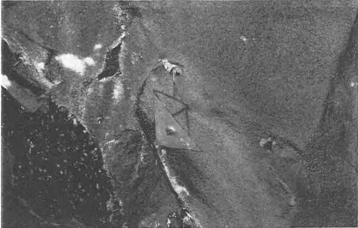
Fig. 3 Stalactites demonstrating leaching of the concrete
